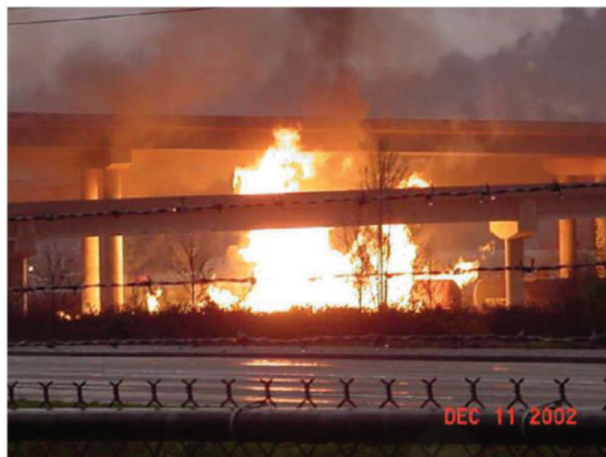
Figure 3.1 Railroad tanker bridge fire in Washington State (Stoddard, 2004).
