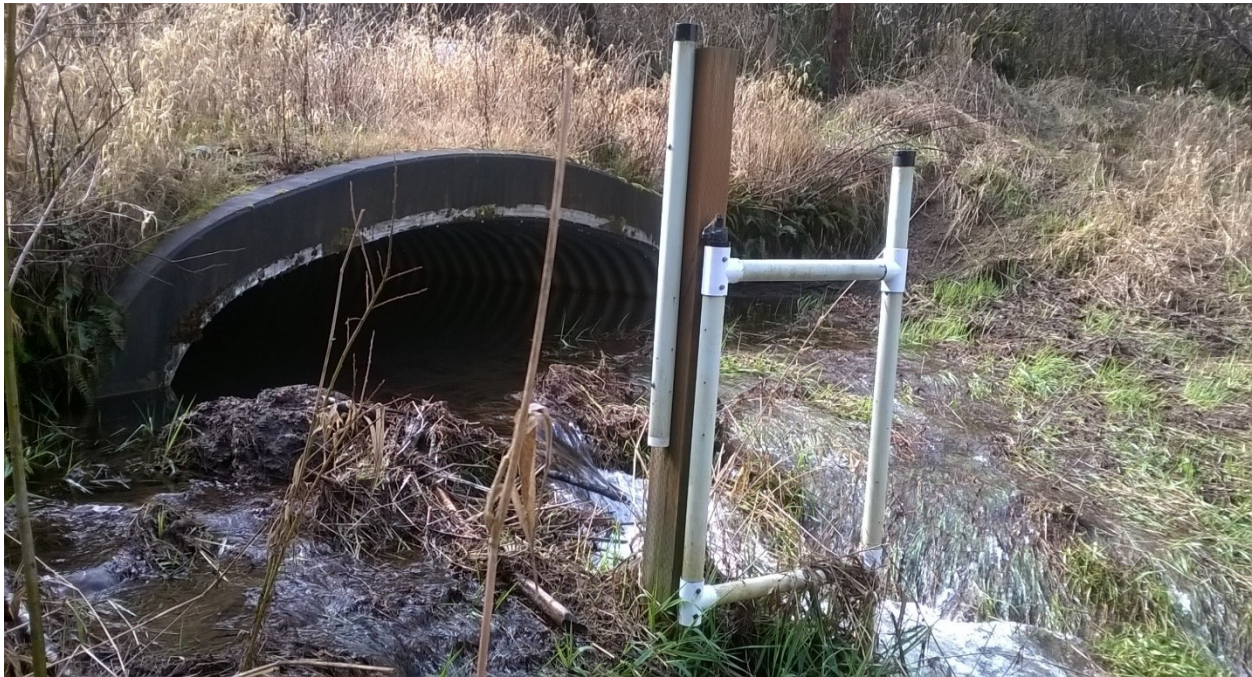
Figure 3.10: Photograph of the station at the Rowdy Creek Culvert showing the Beaver dam that was built and changed normal flow conditions. Photograph taken looking upstream, facing southwest.
