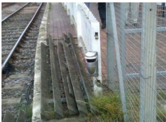
Figure 3-9 Trespasser detection – track surveillance with laser beam in United Kingdom
