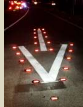
Raised Pavement Markers (RPMs) at Exit Ramp (Source: Provided by Arizona DOT)
