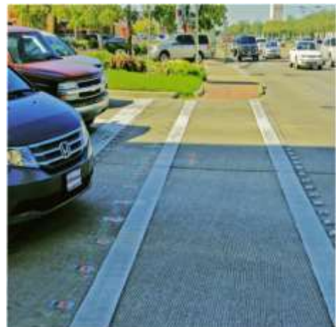
In-pavement LED Lighting at Exit Ramp (Source: Provided by HCTRA)
