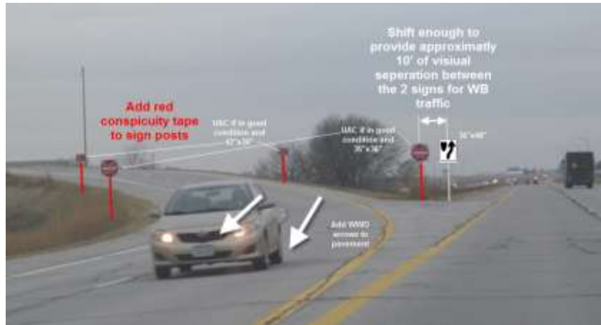
Improvements at Lincoln Way Flyover Ramp: Signs on Both Sides of Ramp, Red Conspicuity Tape on Posts, Wrong-Way Arrows (Source: Iowa DOT)
