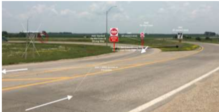
Improvements at 19 th Street Interchange: Stacked DNE and WW Signs on Both Sides, Red Conspicuity Tape on Posts, Wrong-Way Arrows (Source: Iowa DOT)
