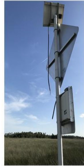
Broken cable at Site 16 (EB, 28°50'07.8"N 82°37'24.6"W)
