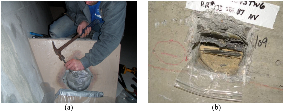
Figure 2-19 Sampling of defective grout in different locations: (a) End cap and (b) Internal tendon (Theryo et al., 2013).
