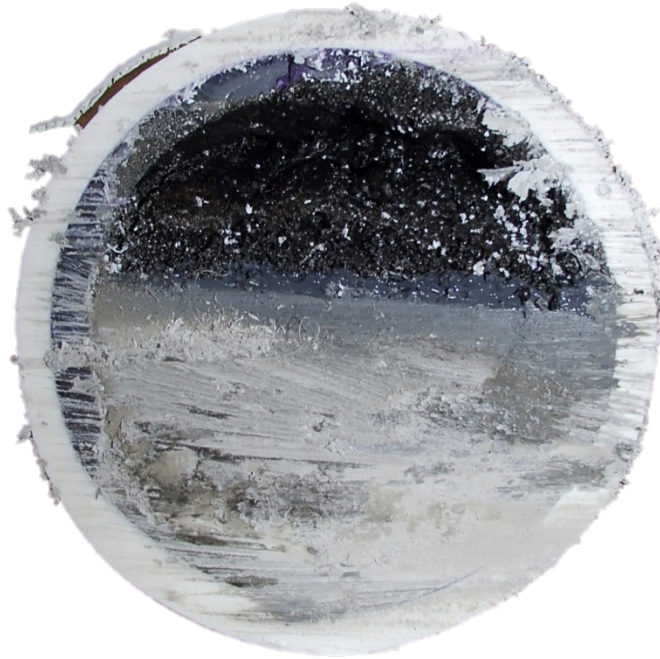
Figure J-13 Cross-section at top of duct where soft grout may be found during MITT
