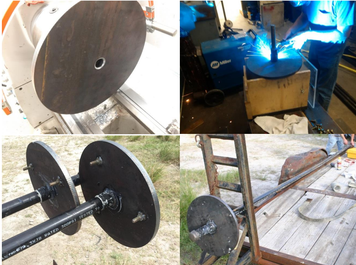
Figure 4.6 One quarter inch chamfer (top left), coupler and nut welded (top right), shear studs to prevent rotation during rod installation (bottom left), and completed anchor bar and base plate assembly (bottom right).
