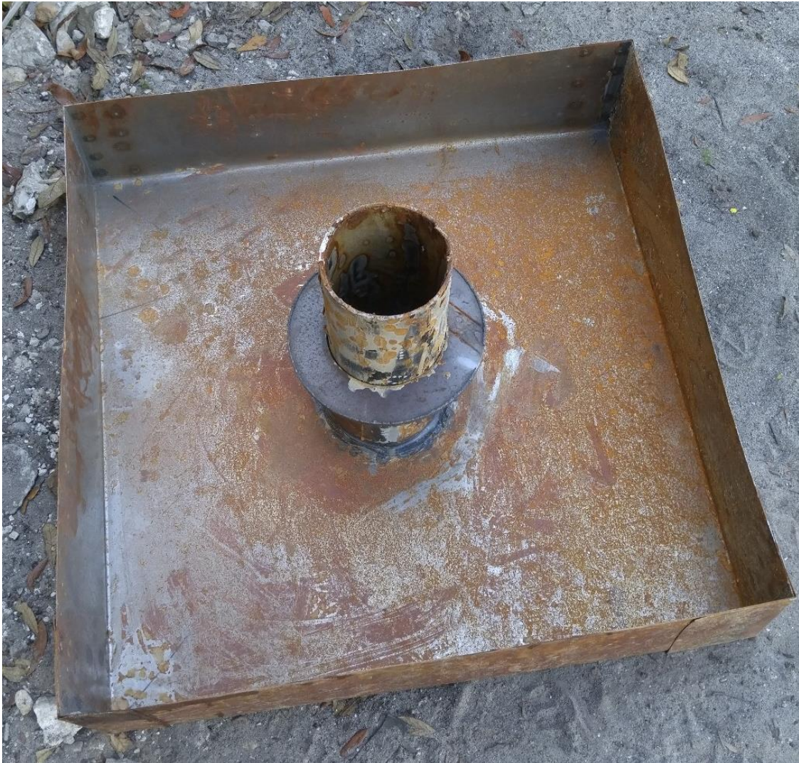
Figure 3.10 slurry catch pan and spill ring installed around casing.
