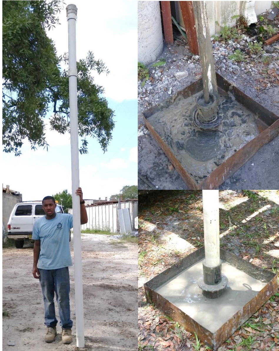
Figure 3.14 Twelve foot long, 3in diameter tremie (left), poor slurry displacement with 2in tremie (top right), improved slurry displacement with 3in tremie (bottom right).
