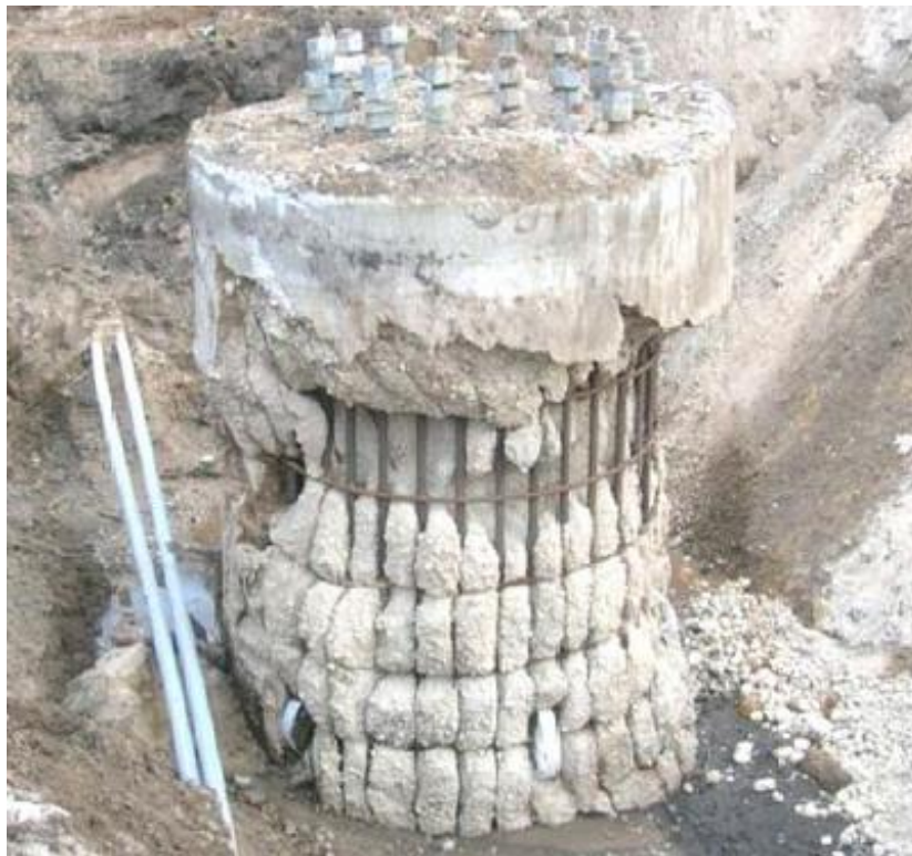
Figure 2.5 exhumed shaft showing poor concrete flow resulting from poor slurry/concrete properties (Mullins et al., 2014).
