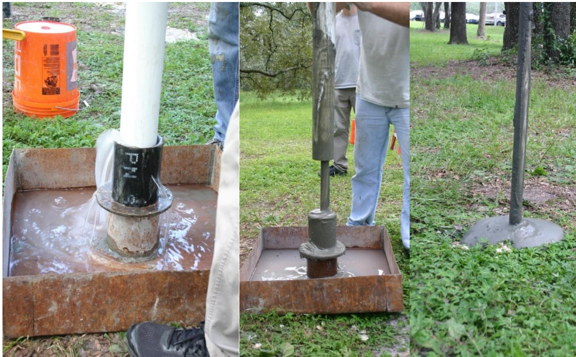
Figure 3.88 Concreting of Cetco polymer shaft; slurry displacement (left), concrete overflow (middle), completed shaft (right).
