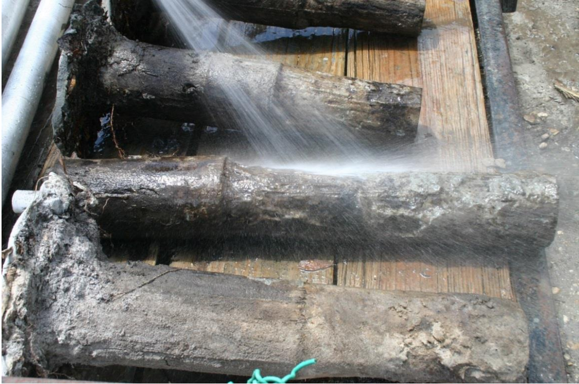
Figure 3.72 Soil bonded to concrete surface in upper 3ft of KB Polymer shafts.
