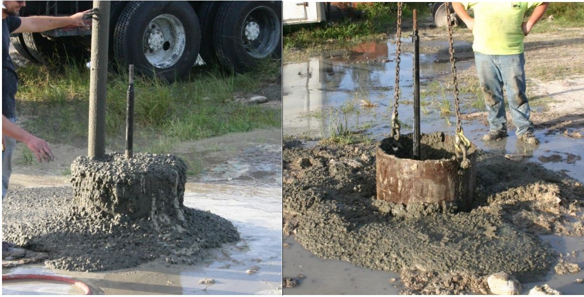
Figure 4.21 Tremie placed aside suspended anchor bar (top left), slurry displacing during concreting (top right), concrete overflow (bottom left), and casing removal (bottom right).
