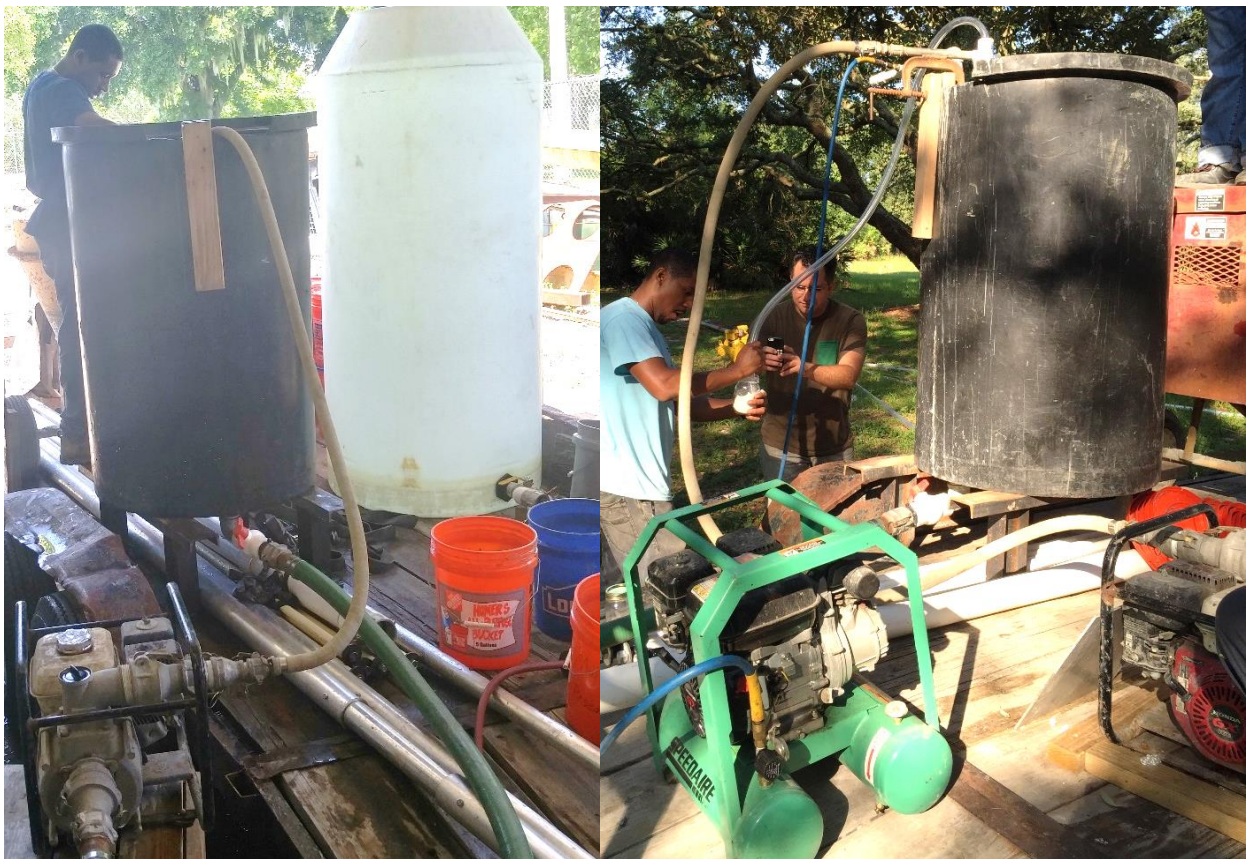
Figure 3.8 Slurry mixing system; re-circulating (left), mixing (right).
