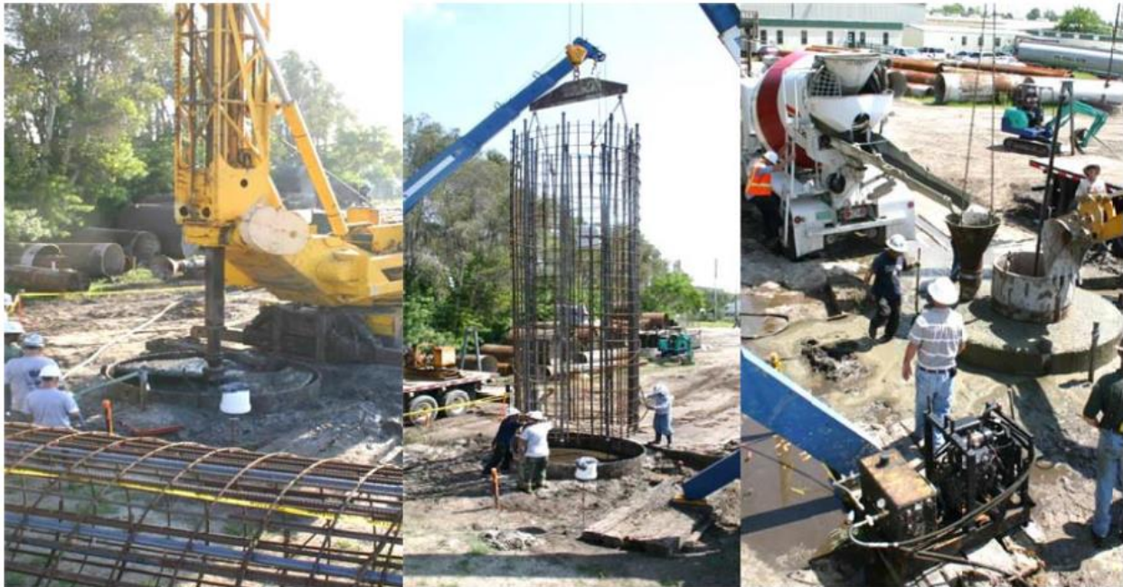
Figure 2.1 Drilled shaft construction: excavation (left), reinforcement cage placement (middle), concreting (right) (Mullins et al., 2014).
