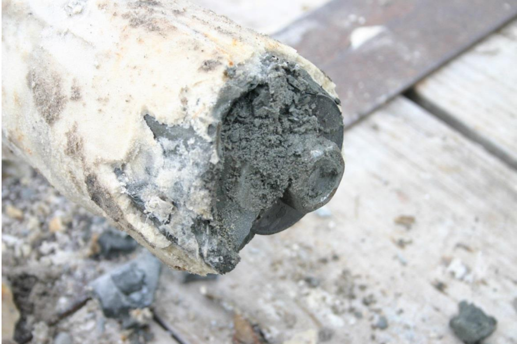
Figure 3.70 Moisture laden mortar at the base of the shaft.
