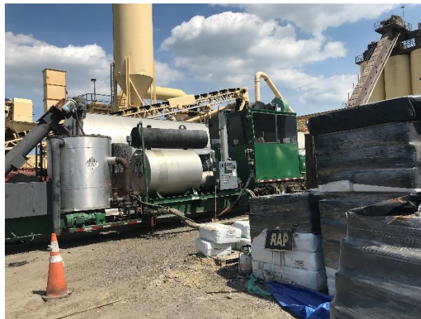
Figure 6. GTR and Asphalt Binder Mixing Tank to the Left and System Control House to the Right. GTR = ground tire rubber.
