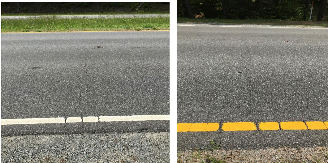
Figure 10. Reflective Cracking Observed on US 60 After 2 Years
