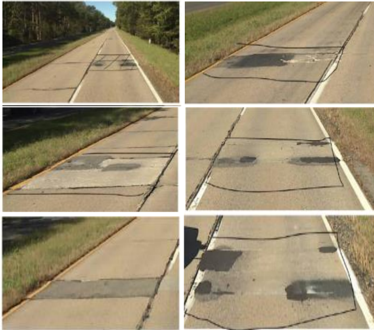
Figure 2. Existing Pavement Distress on US 60 (New Kent County)
