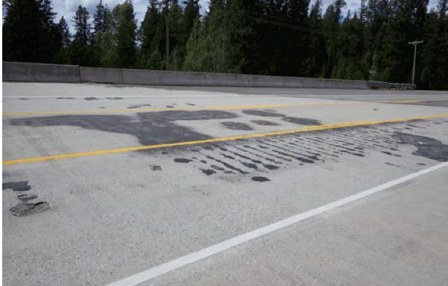
Figure 3. Large Area of Concrete Spalls with Rebar Exposed and Delamination at Midspan of the Deck
