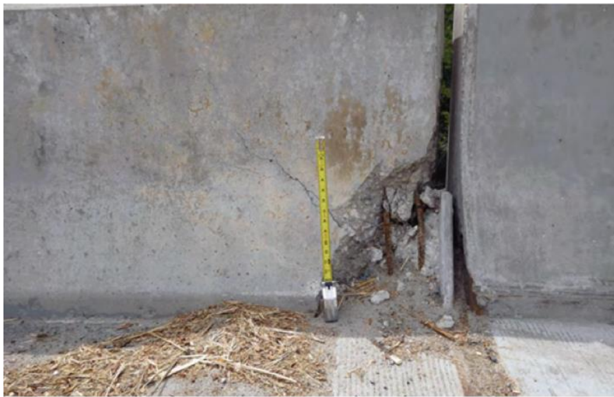
Figure 4. Concrete Spalling in a Concrete Rail (District 1)
