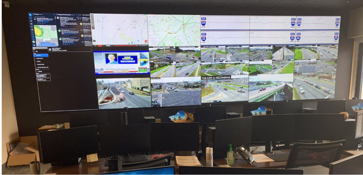
Figure 9 West Central RTMC speed dashboard (upper right) in existing ATMS
