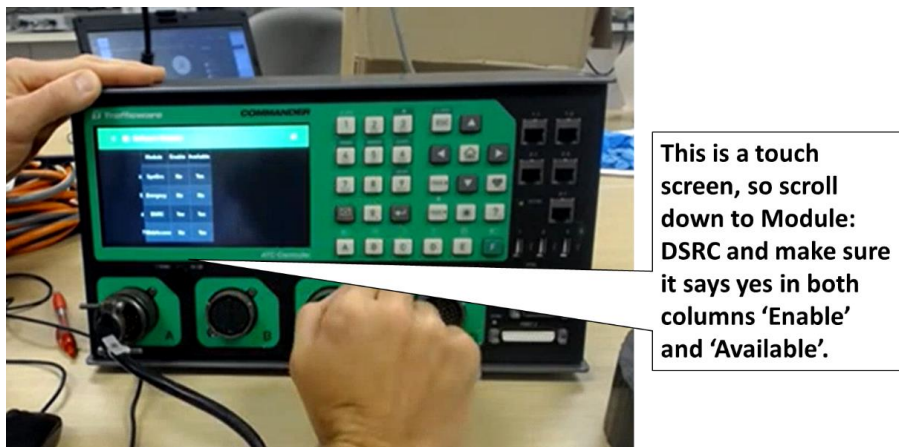
Figure 7. Trafficware Commander Initializing Controller- Scroll to DSRC
