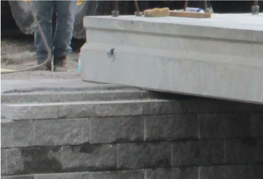
Figure 20 Bridge beam setting on top of CMU with 3-in gap between abutment and beam and integrated approach reinforcement layer. The circular opening for post-tensioning can be seen at the end of the beam.
