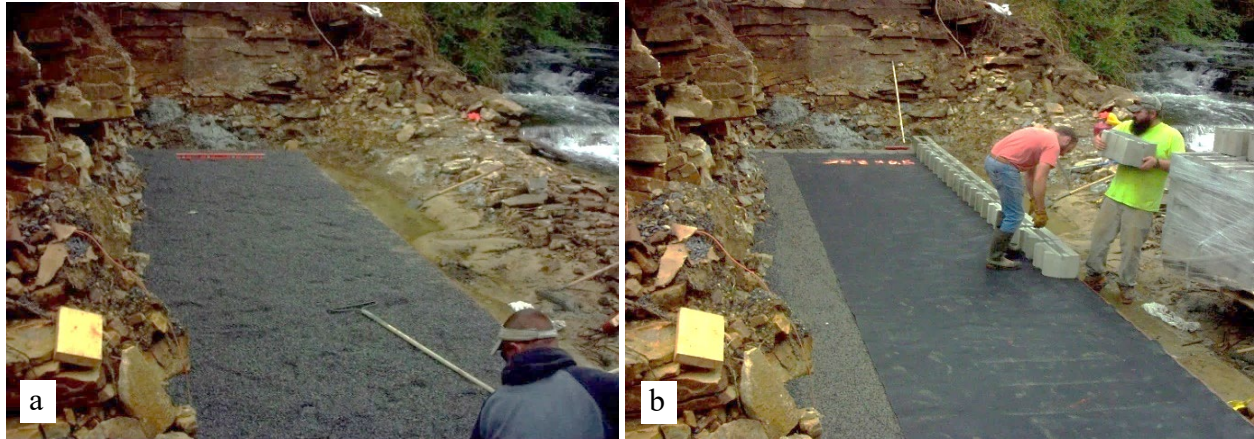
Figure 18 Placement of initial layer of No. 89 stone to top of first row of masonry blocks and (b) placement of geosynthetic and second row of masonry blocks.
