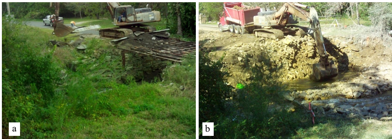
Figure 16 (a) Removal of the existing bridge at Turkey Creek; (b) removal of blasted sandstone, on the western side of Turkey Creek.
