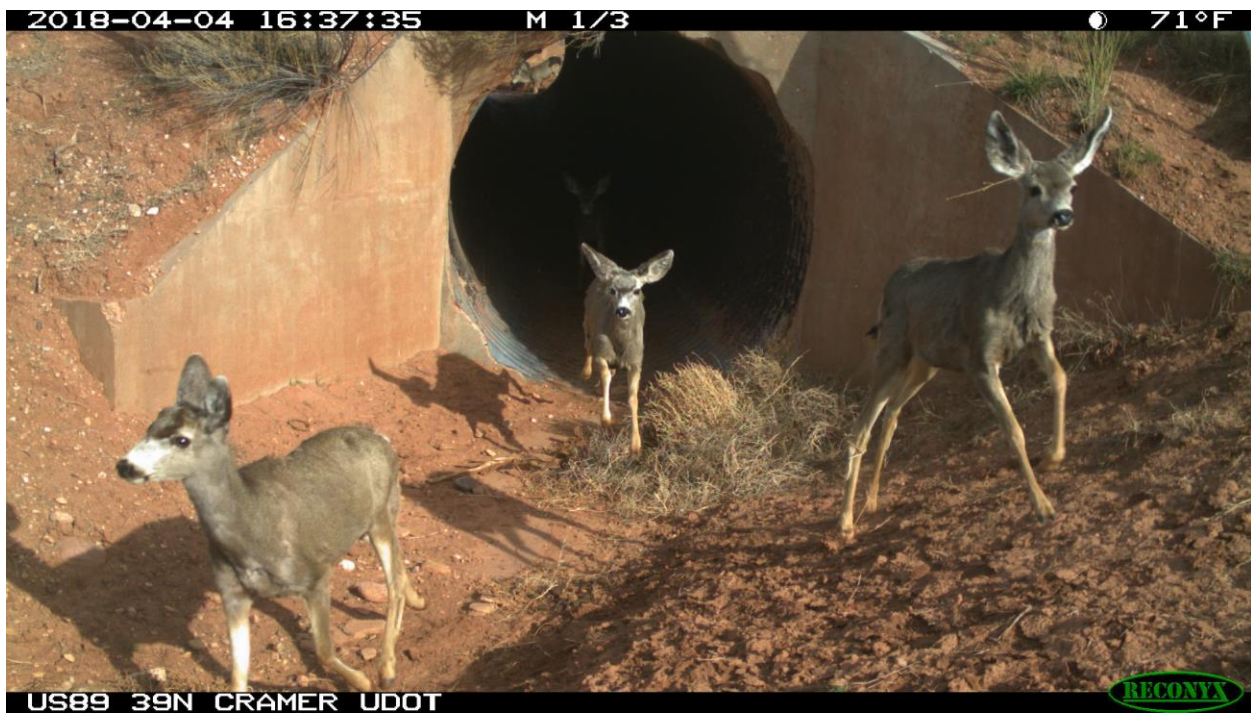
Mule Deer Moved Through the Telegraph Culvert from the South in the 2018 Spring Migration.
