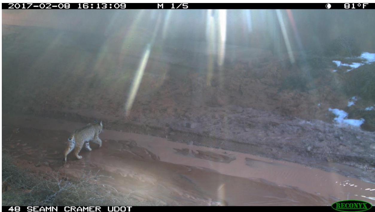
Bobcat Used Seaman Culvert, February 2017.
