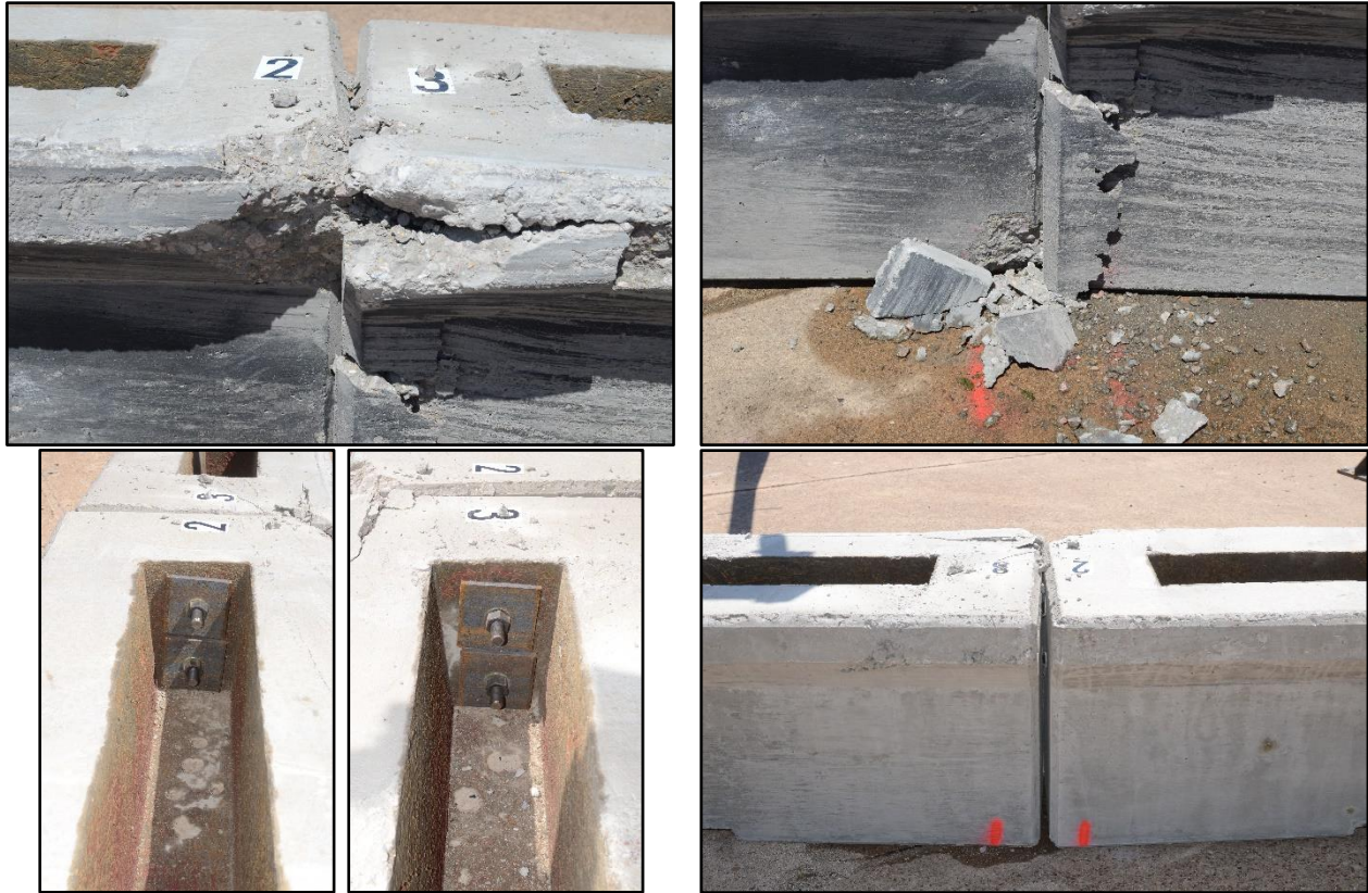
Figure 7.4. Damage at Joint 2-3 after Test No. 469688-1-2.
