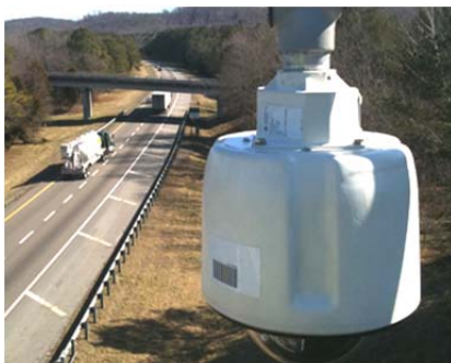
Figure TN-2. CCTV camera.
