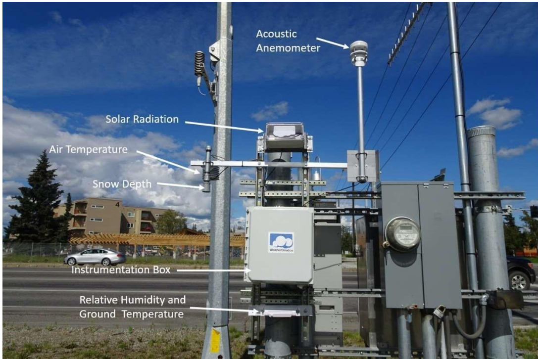
Figure 3.1 Cowles Street installation
