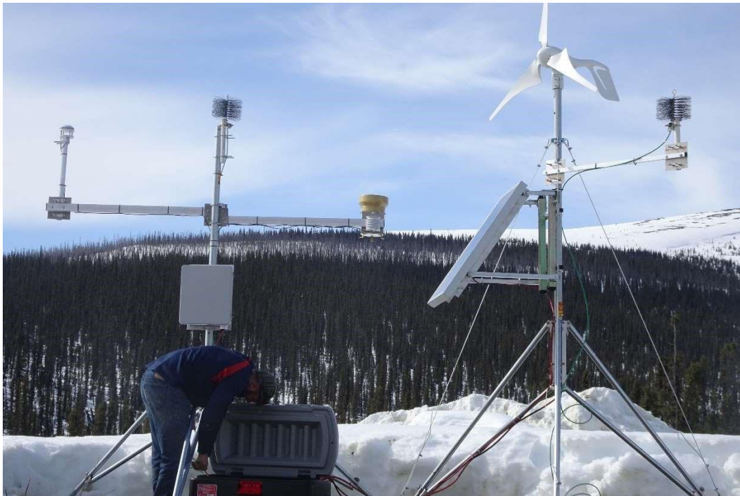
Figure 7.1 Montana Creek installation
