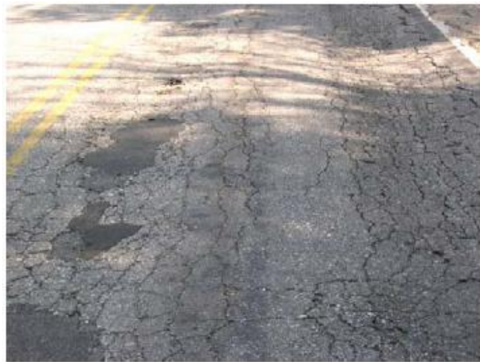
Figure 3.10 Example of alligator cracking, heavy severity.
