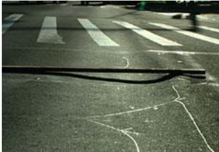
Figure 3.19 Example of rutting, high severity
