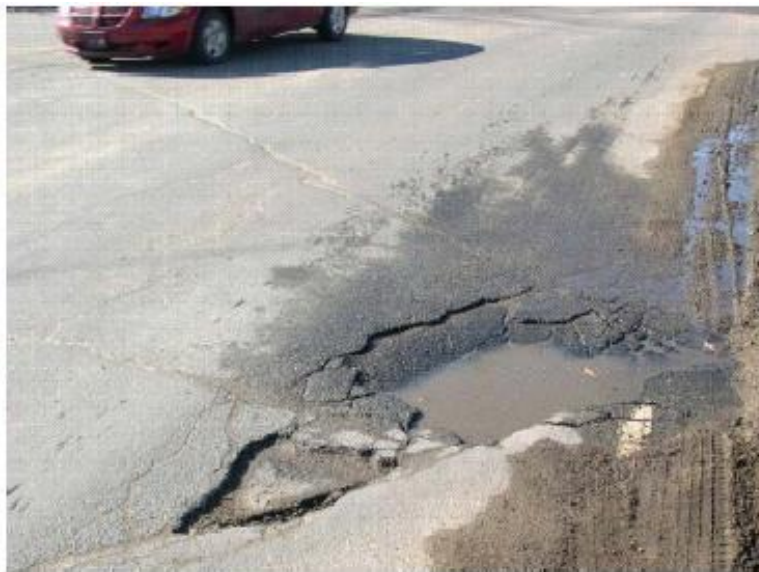
Figure 3.16 Example of potholes, high severity
