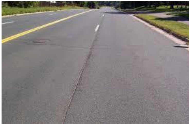
Figure 3.18 Example of rutting, medium severity
