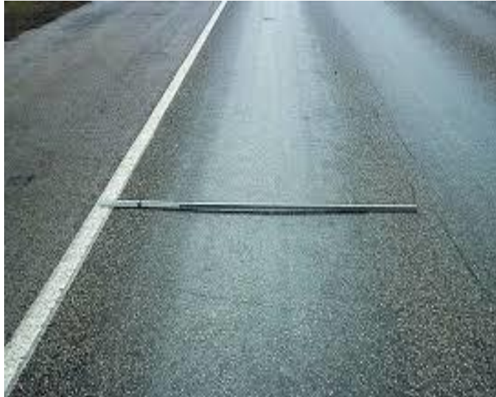
Figure 3.17 Example of rutting, low severity
