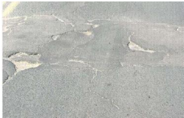
Figure 3.14 Example of potholes, slight severity
