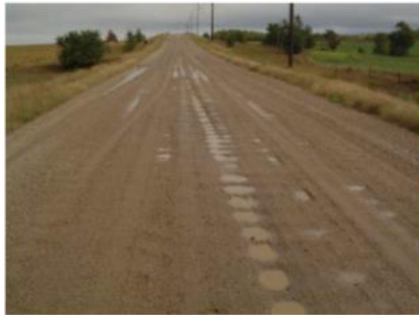
Figure 3.21 Gravel road with inadequate crown
