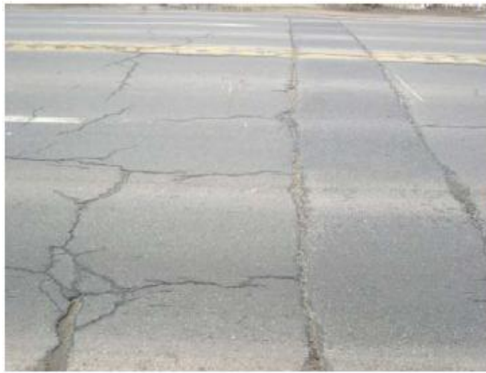
Figure 3.12 Example of block cracking, moderate severity.
