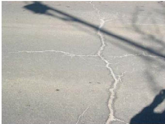
Figure 3.6 Example of longitudinal and transverse cracking, medium severity.
