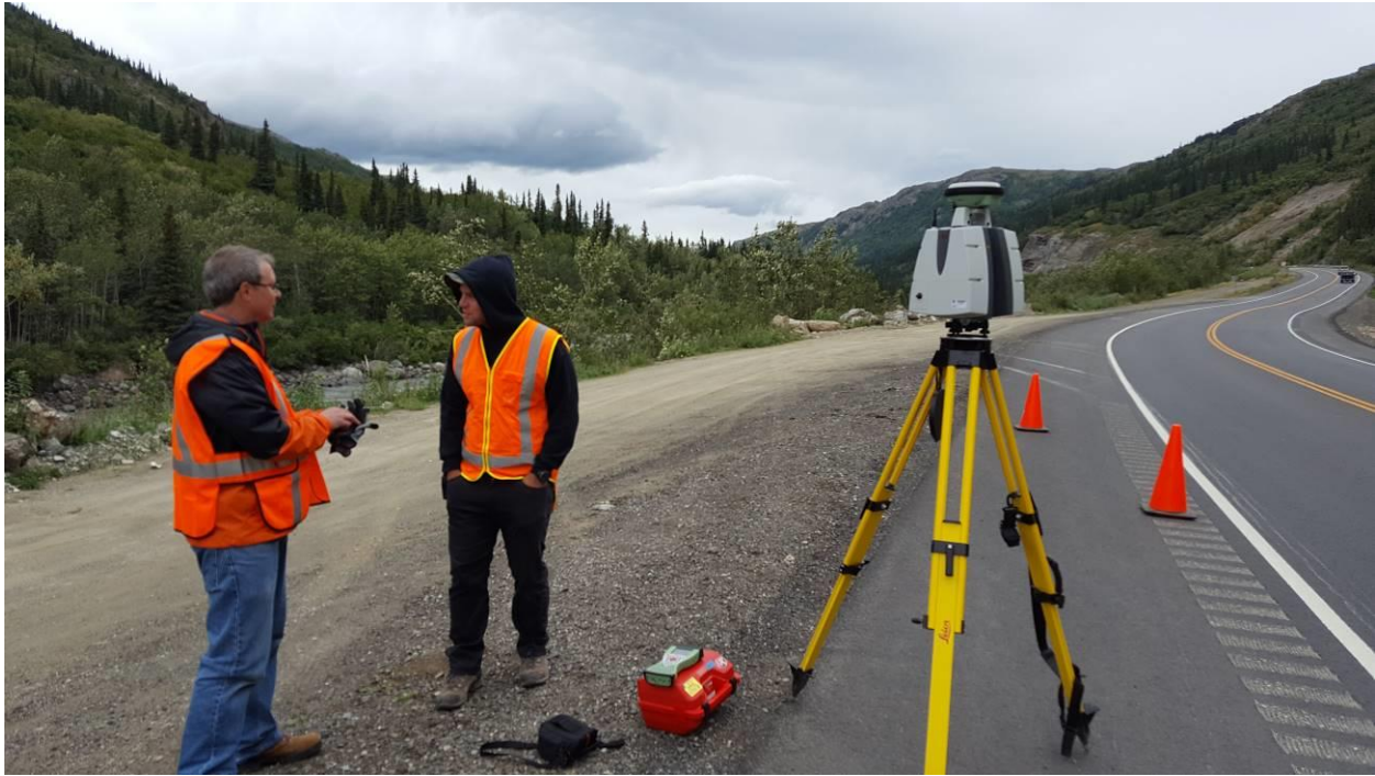
Figure 4.2 Example terrestrial laser scan set-up with the Leica P40 at a Glitter Gulch site.
