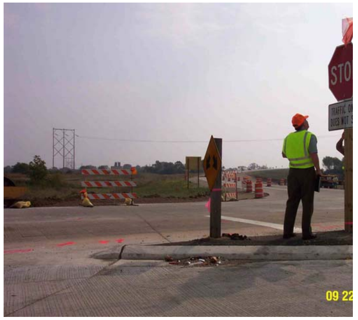
Picture 17 – at STH 89 north of US 12 @ ~8' behind stop bar right turn lane (kneeling to approximate driver eye height) looking East on USH 12
