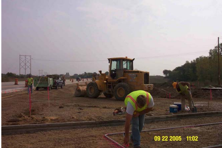
Picture 18 – on STH 89 South of US 12 @ ~8’ behind stop bar (kneeling to approximate driver eye height) looking East on USH 12
