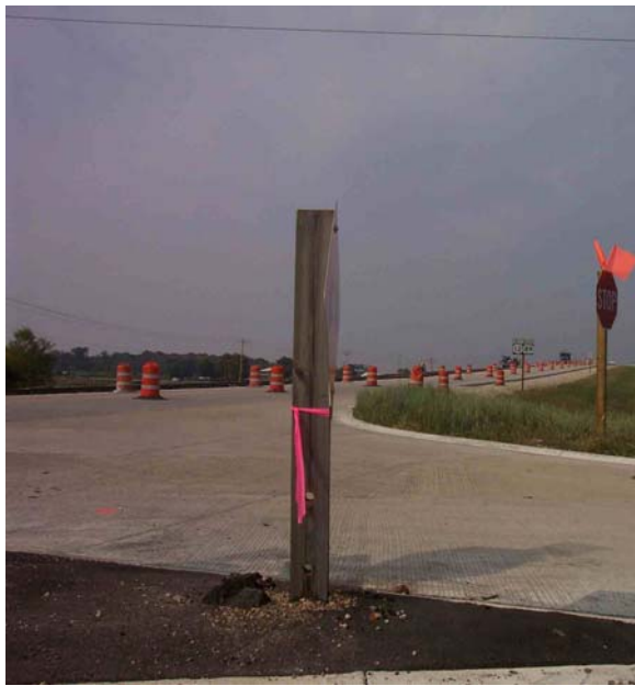
Picture 16 - at STH 89 north of US 12 @ ~8' behind stop bar left turn lane (kneeling to approximate driver eye height) – looking West on USH 12
