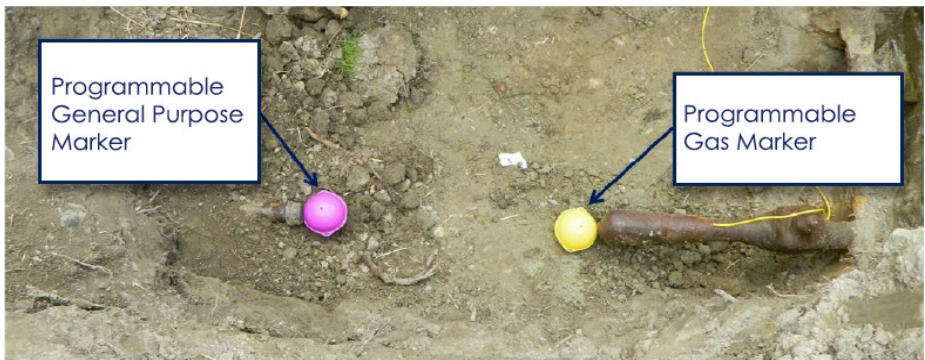
Figure 1. Marker balls give a robust point-to-point picture of newly installed utilities and allow personnel to “connect-the-dots” with fairly accurate results using readily available RFID software technology.
