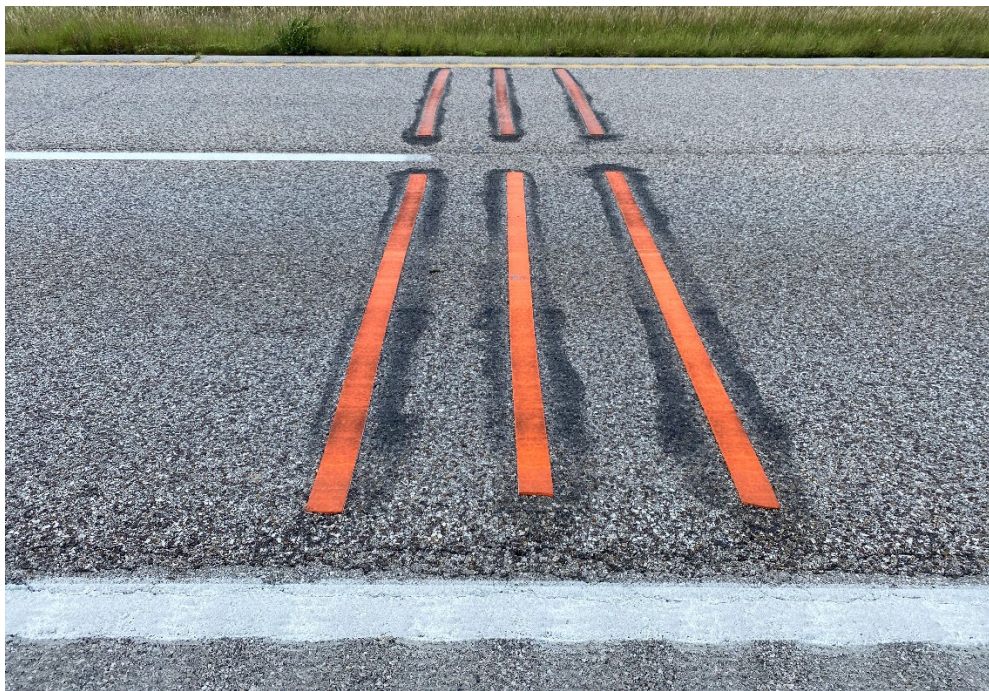
Figure 5-6. Long-term temporary rumble strips on I-55 in Ste. Genevieve County
