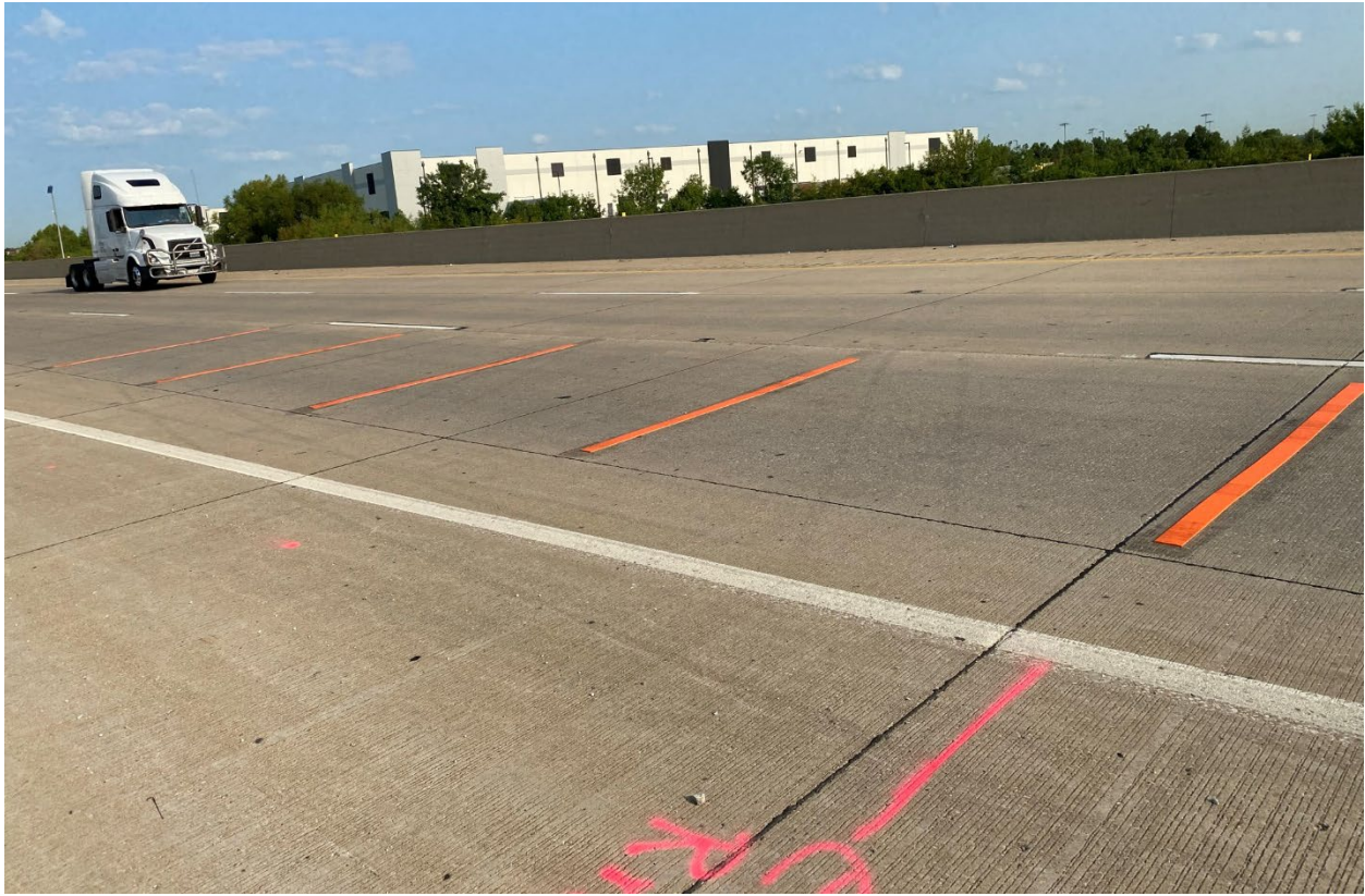
Figure 5-4. Long-term temporary rumble strips on MO 370 in St. Charles County
