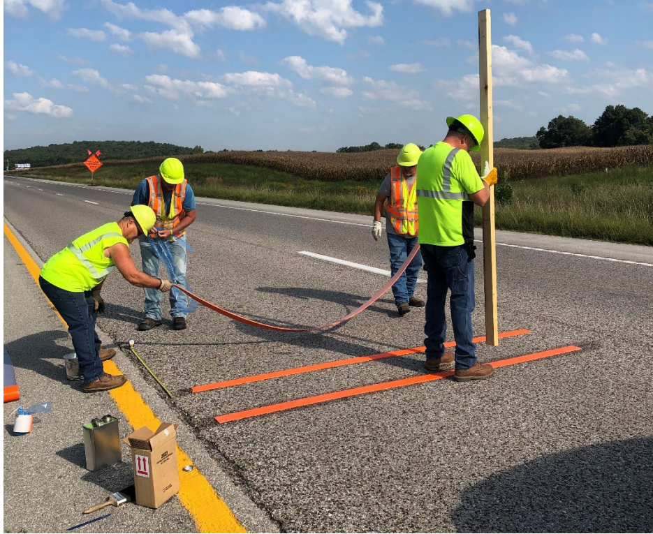
Figure 5-5. Placement of long-term temporary rumble strips on I-55 in Ste. Genevieve County
