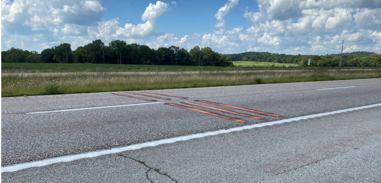
Figure 4-3. Temporary rumble strips on I-55 in Ste. Genevieve County
