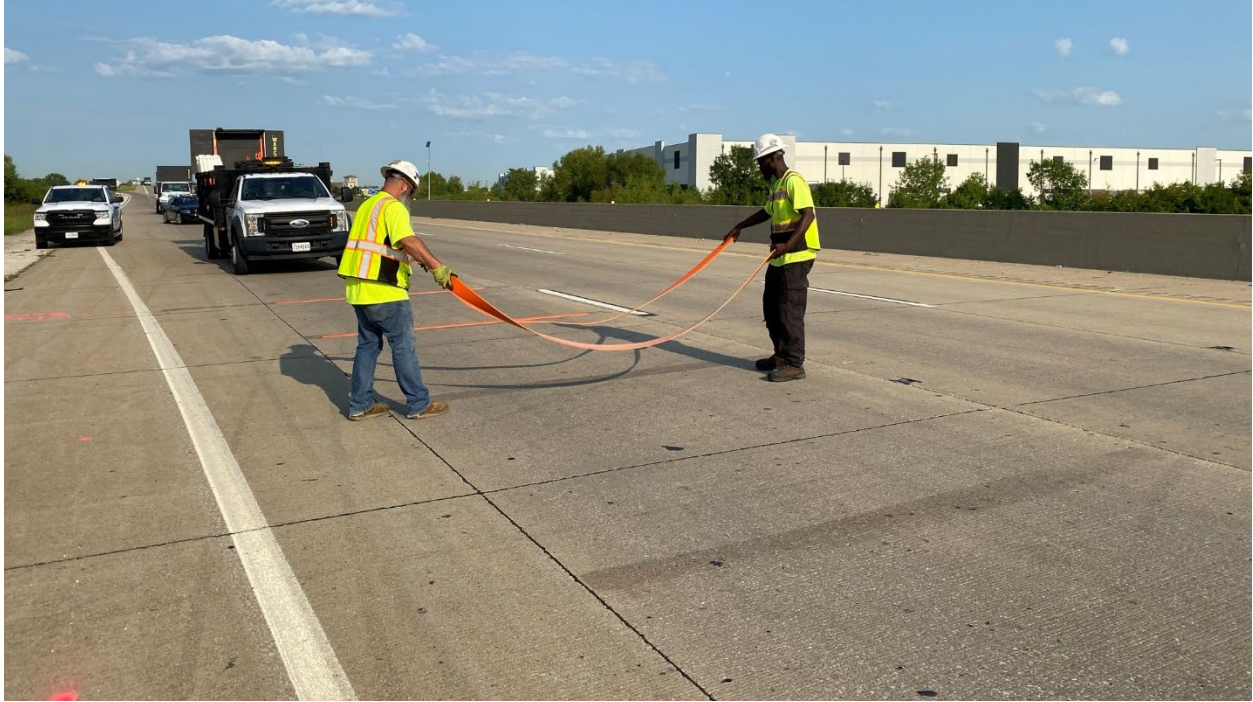
Figure 5-3. Installation of long-term temporary rumble strips on MO 370 in St. Charles County
