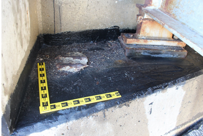
Figure 23. Example of a concrete coating applied to beam shelf under expansion joint to protect concrete substructure, Fulton, MO.
