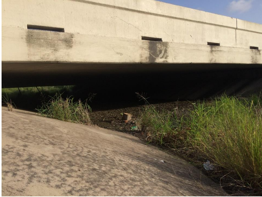
Figure H.2: Photo Taken by P. Cramer under US 48 of the Ocelot Crossing Bridge Structure.
