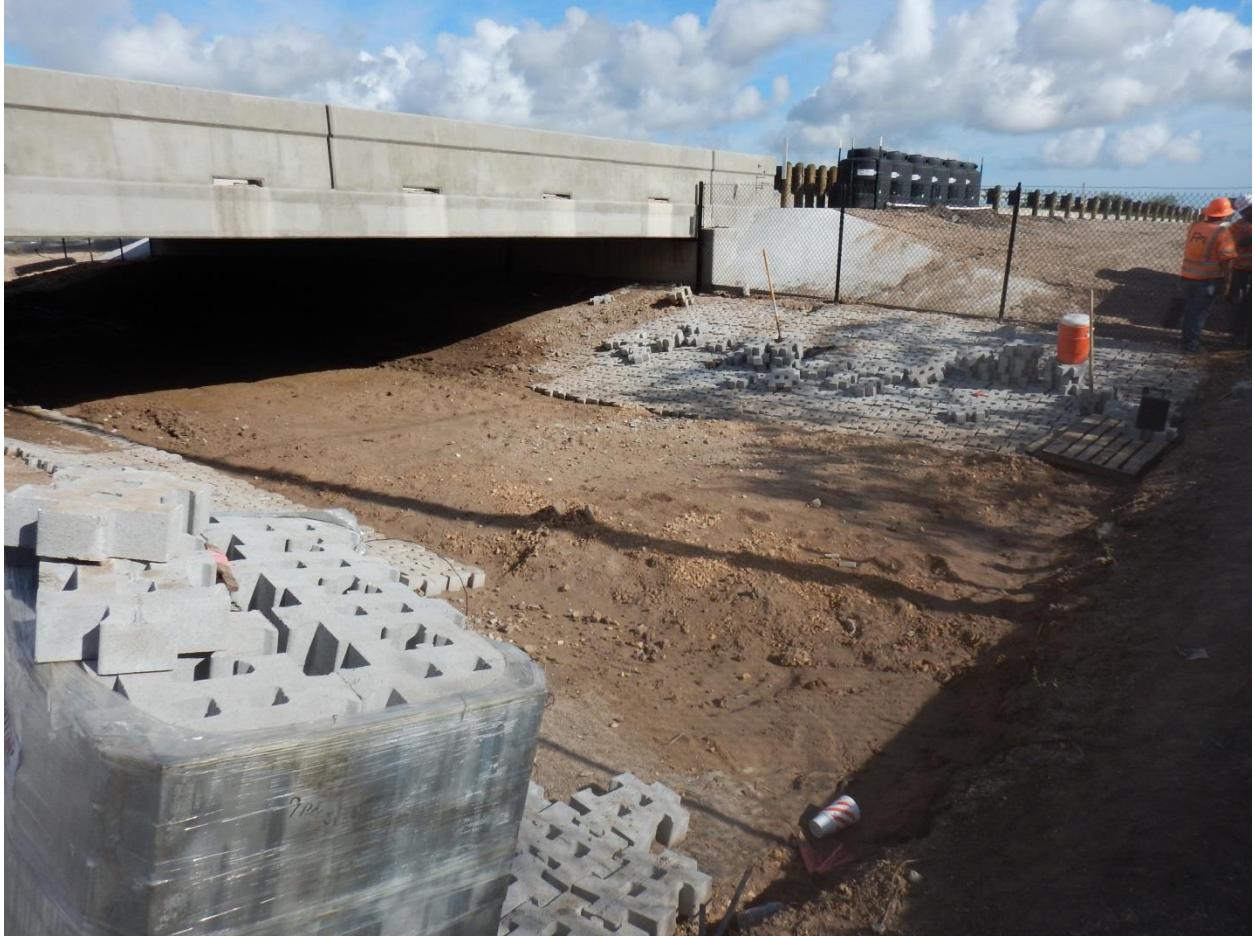
Figure H.14: Half Bridge with the Articulated Mat being placed on SH 100.
