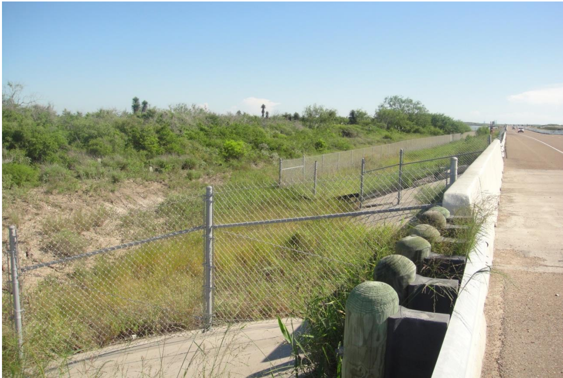
Figure H.1: Photo from on Top of the Bridge Crossing on SH 48, Looking Southwest
