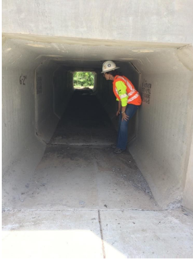
Figure H.10: Terrestrial Box Culvert for Ocelot and Other Species, SH100
