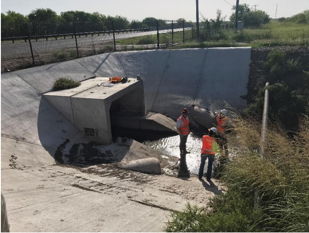
Figure H.8: Photo of FM100 Wildlife Crossing Box Culvert (with Ledges Increasing Access for Animals to Structure)
