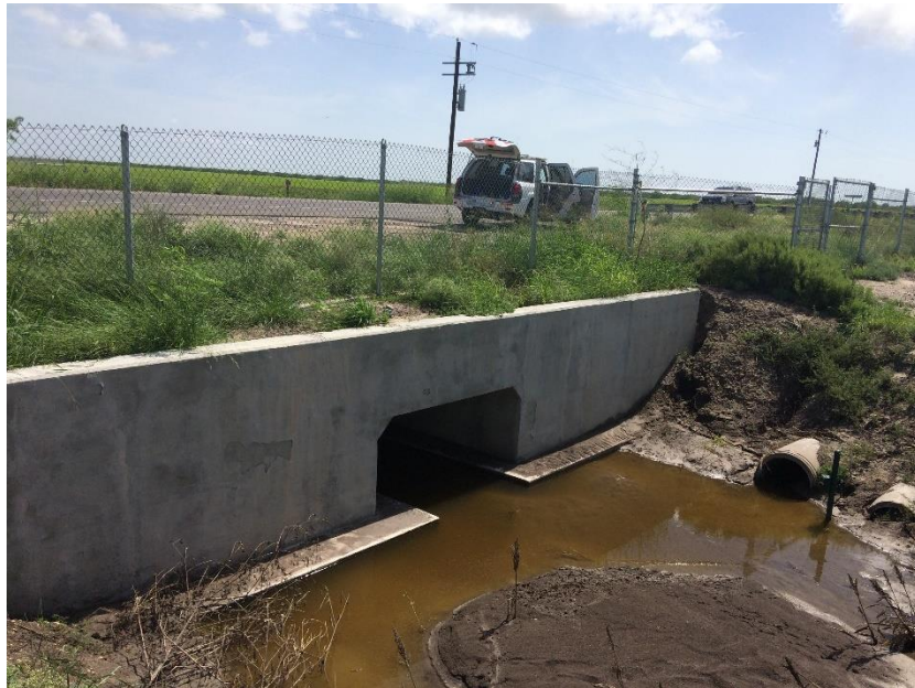
Figure H.9: FM106 Second Structure with Slightly Different Ramp Design (Note: small alligator was seen here.)
