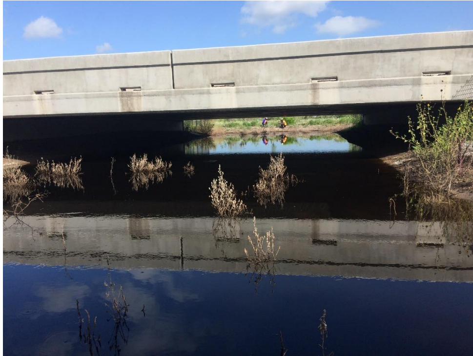
Figure H.15: SH100 Bridge for Wildlife, with Students Checking Cameras on Opposite Side, after a flood event
