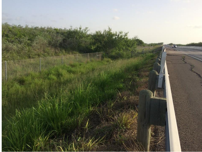
Figure H.18: SH 48 Ocelot Crossing Structure with Chain Link Fence and Guard Rail
