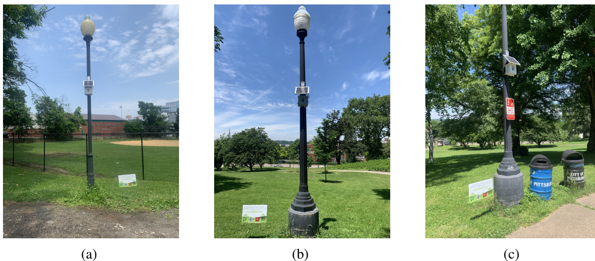
FIGURE 8: Examples of three of the eight sensing nodes installed at (a) Location 1, (b) Location 3, and (c) location 6.
