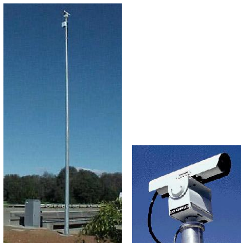
Figure 5. Rural Surveillance Camera Installation
