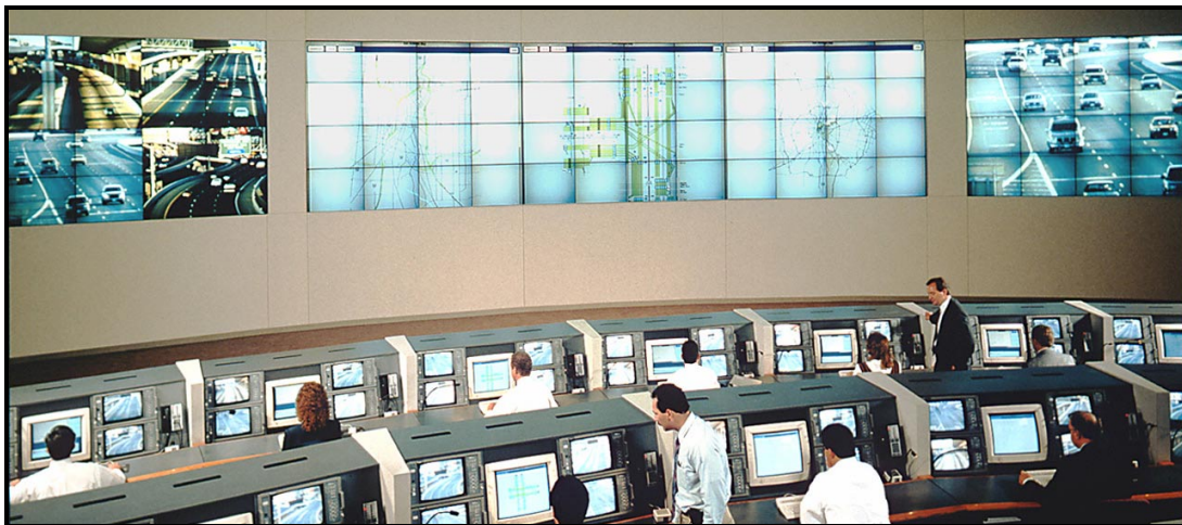
Figure 4. TransGuide System Control Center ( 23 )
