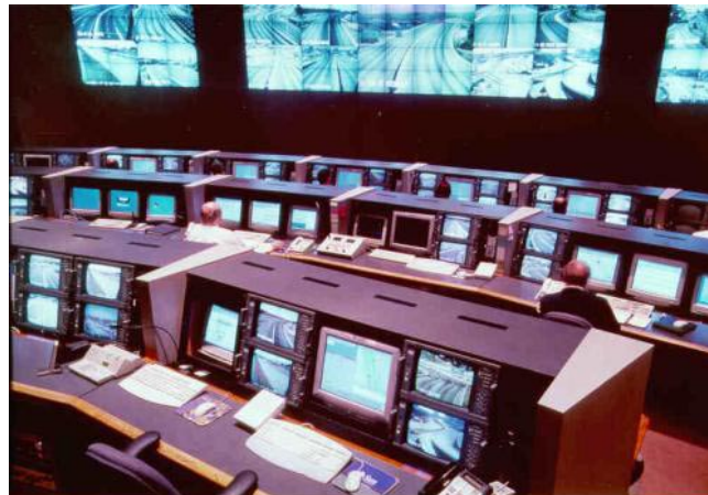
Figure 3. The Control Room of TransGuide in San Antonio, TX
