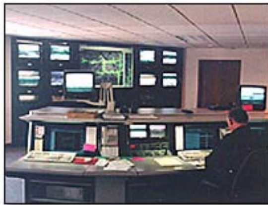
Figure 2. The Control Room of Monitor in Milwaukee, Wisconsin
