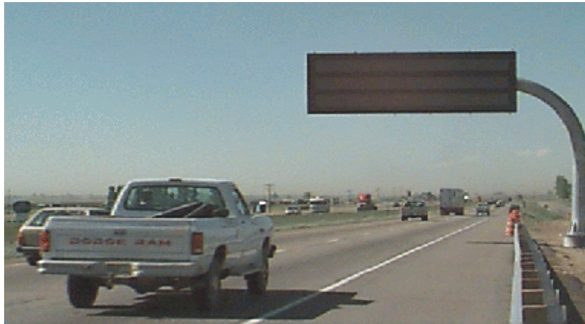
Figure 4. Cantilever Overhead Mounted Dynamic Message Sign
