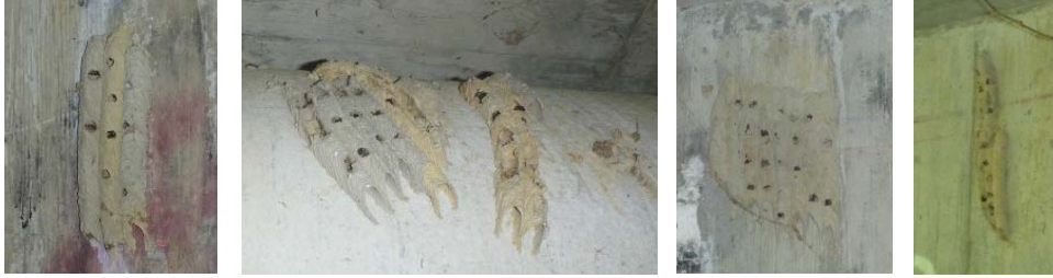
Figure 5-31: Mud-Dauber's nests observed at MA-concrete
