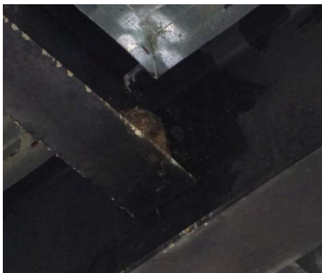
Figure 5-69: Bird's nest at NH-steel_truss
