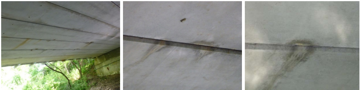
Figure 5-37: Staining in between beams in MA-precast_concrete
