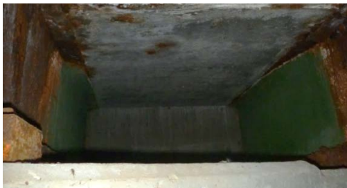
Figure 5-50: Cave-like environments near the abutments at MA-steel
