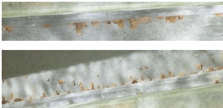
Figure 5-76: Mud-Dauber's nests observed on girders of RI-concrete
