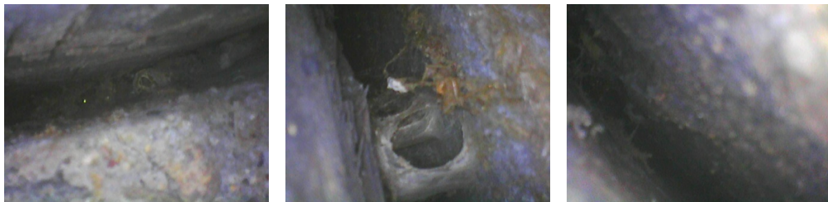
Figure 5-28: Boroscope views of crevices in MA-concrete
