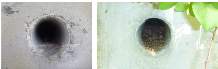
Figure 5-75: Drainage features observed in RI-concrete
