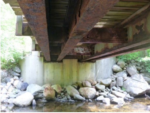
Figure 5-20: Significant deterioration and staining in ME-steel/wood
