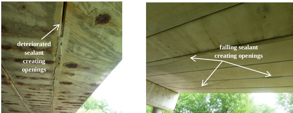
Figure 3-7: Deterioration of the sealed gaps between beams
