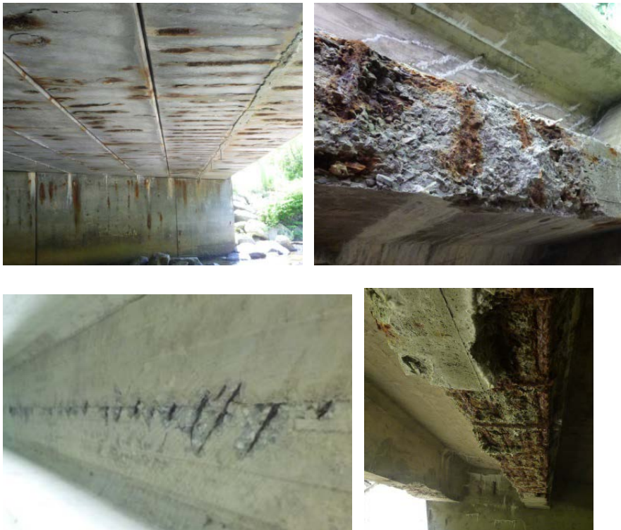
Figure 3-11: Not all deterioration will create crevices
