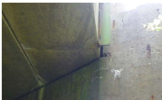
Figure 5-40: Gaps under beams at MA-precast_concrete_2
