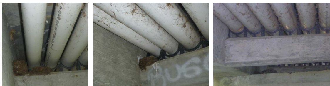
Figure 5-30: Birds' nests and pipes observed at MA-concrete
