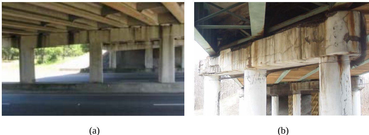
Figure 4-16: Photo of staining observed on a bridge pier shown in the federal report intended to demonstrate the ‘staining’ indicator on the federal form (photos courtesy of Jeff Gore, Florida Fish and Wildlife Conservation Commission) (a) and typical deterioration staining on a New England bridge pier slated for construction (b)
