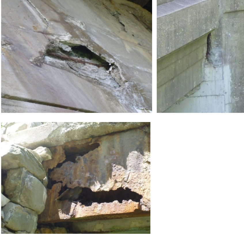
Figure 3-10: Localized deterioration creating suitable roosting crevices
