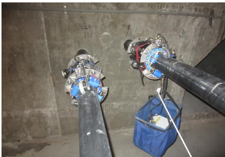
Figure 15. Two permanent magnet type MMFM magnetizers installed on PT tendons.
