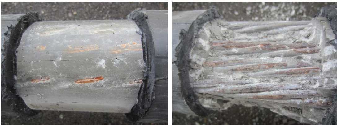
Figure 45. Back face of the suspected damage area as exposed (left) and after grout layer was partially removed (right).
