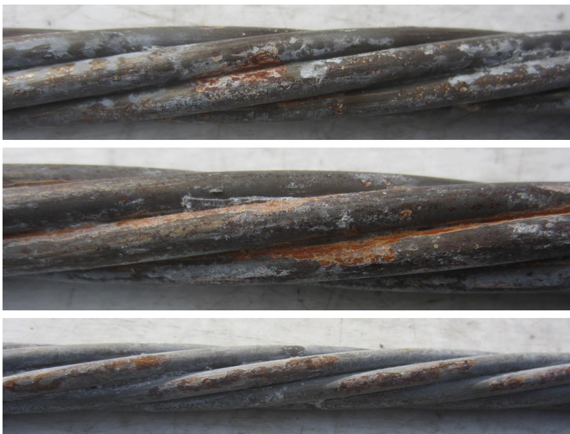
Figure 48. Representative conditions of rusted strands.
