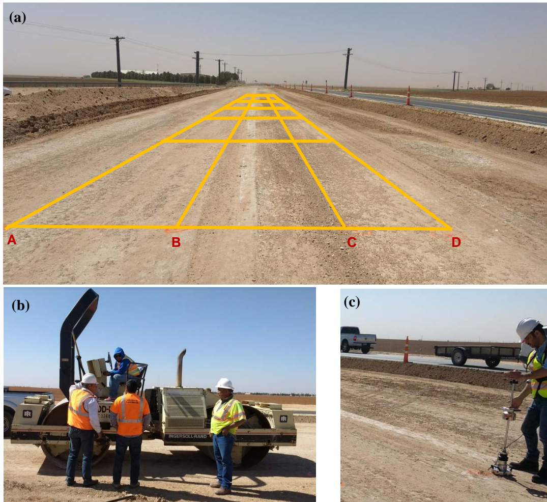
Figure K.3 – (a) Test Section, (b) Instrumentation of Roller Compactor with Data Acquisition System and Recommendations Provided to Roller Operator and (c) Deflection-Based Spot Testing using the LWD.
