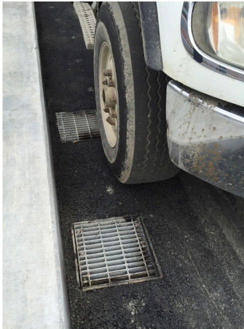
Figure 14 – FRP drains in service (2015-06-03)
