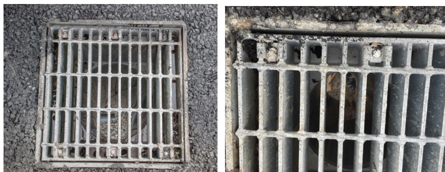
Figure 13 – a) Drain top and grate; b) Detail showing condition of the FRP scupper wall (2015-06-03)
