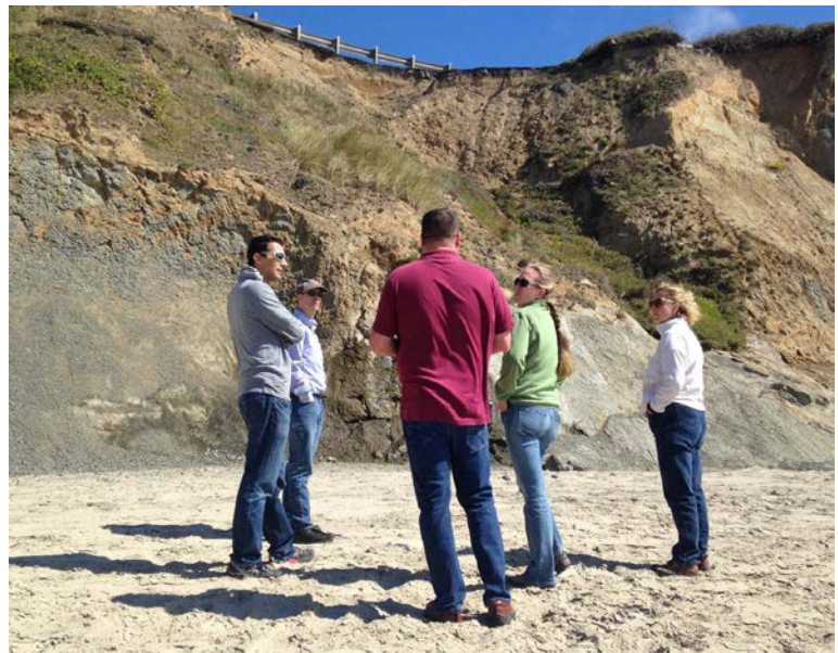
The ODOT team met with FHWA representatives to discuss erosion issues at Beverly Beach. Credit: ODOT.
