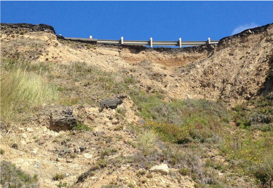
Wave action from storms has eroded away areas of roadway asphalt and is close to compromising the guardrail along US 101, southbound lane. Credit: ODOT.
