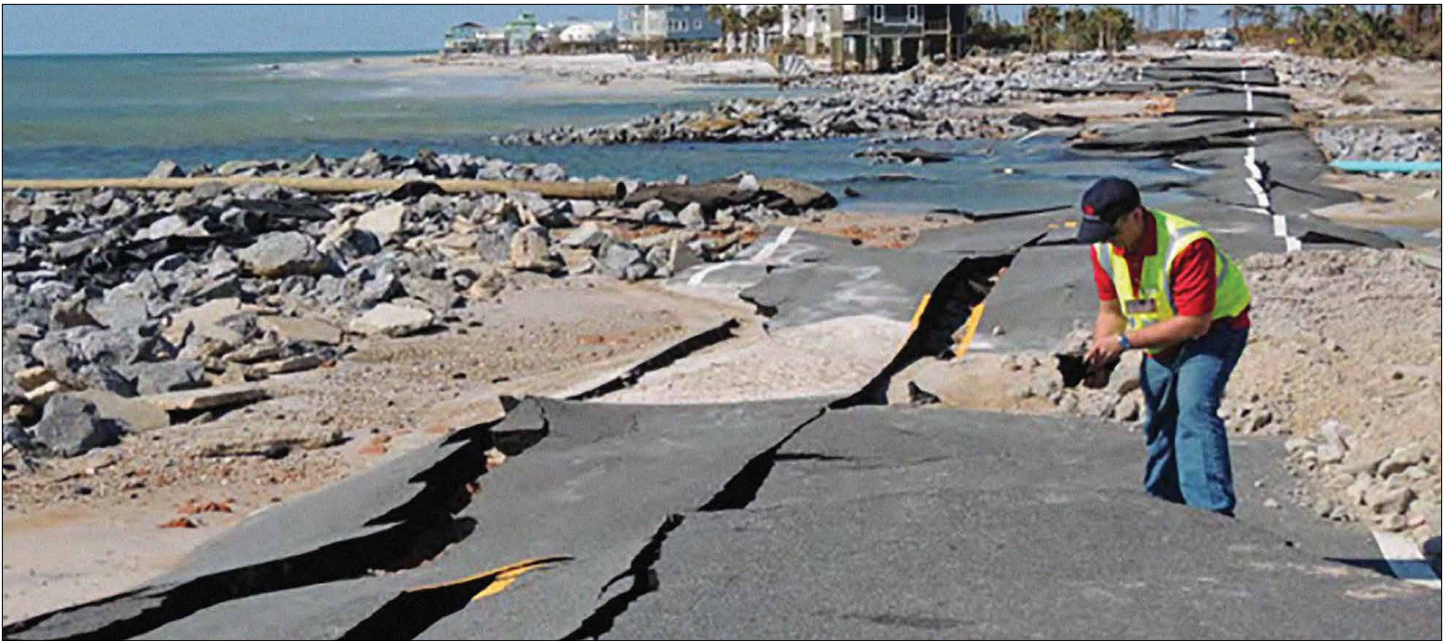
Example of roadway impacts and pavement damage from coastal hazards. Photo: FHWA-HIF-19-059 January 2020 Hydraulic Engineering Circular No. 25
