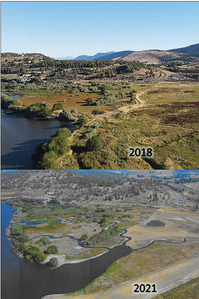
Before and after images in the dry season showing the construction of channels and pond, as well as the removal of the contaminated dike. Photos: Oregon Department of Transportation
