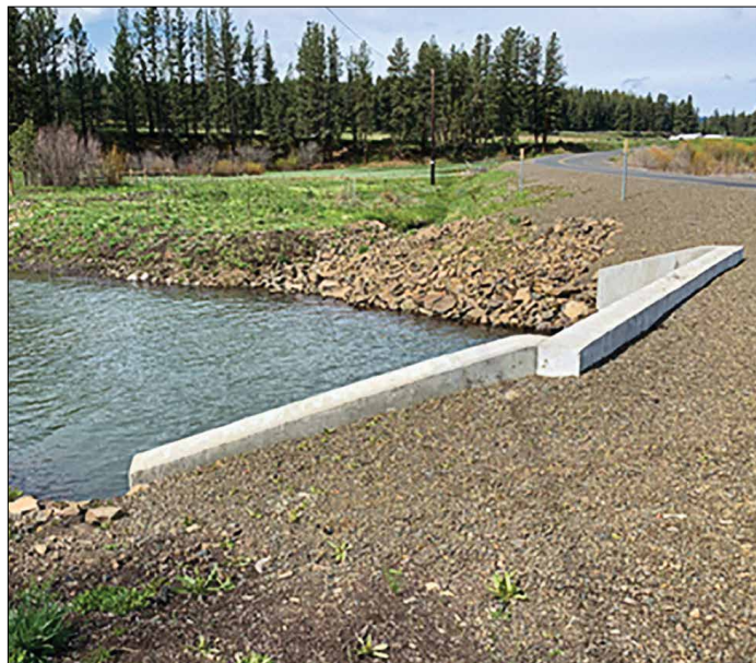
The replacement of the Whiskey Creek culvert with a 22-foot-wide, pre-cast reinforced concrete box culvert. Photo: Oregon Department of Transportation
