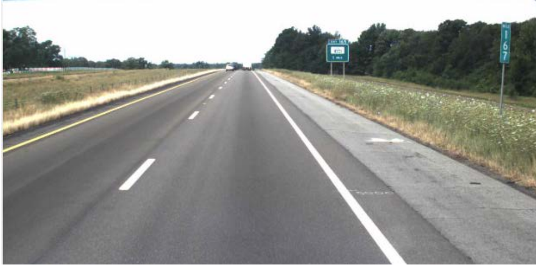
Figure 104. IH 30 Westbound Area with Deep Rutting.
