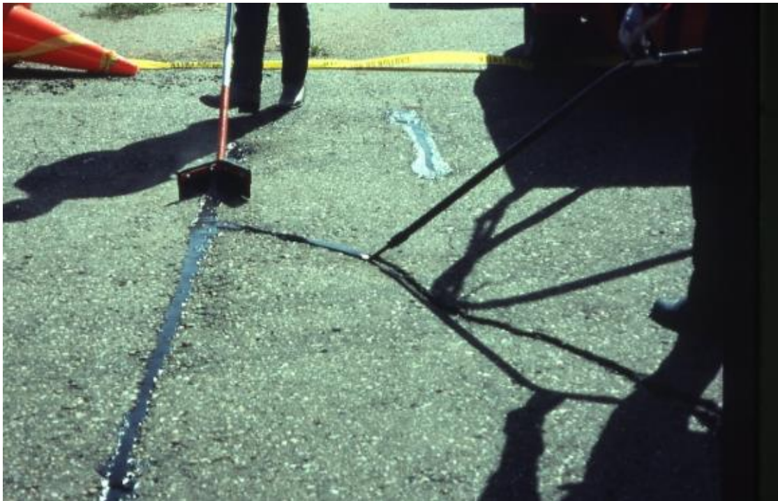
Figure 13. “Flush fill” of Crack
