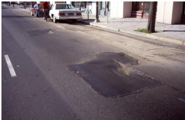
Figure 46. Weak, Unstable Asphalt Mix Used in Patches on a City Bus Lane
