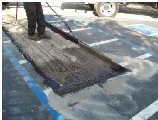
Figure 36. Cut the Boundaries of the Patch and Tack Coat on Vertical “cut” Edges
