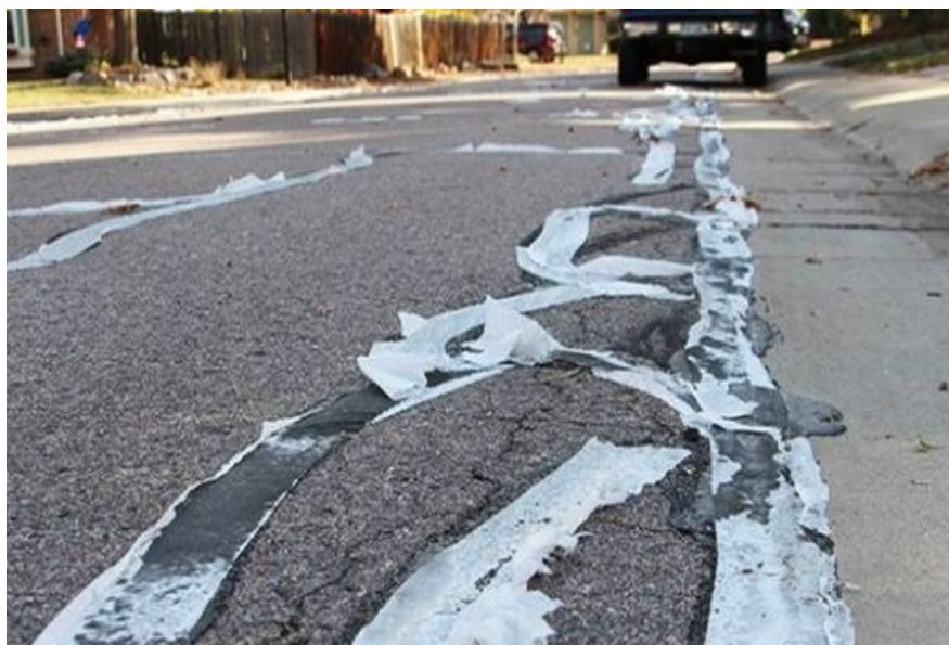
Figure 23. Improper Blotting Techniques Using Paper
