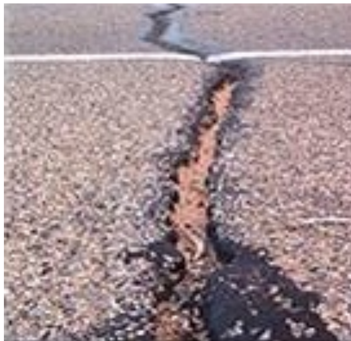
Figure 11. Example of a Badly Cleaned Crack (Courtesy of Crafc0)
