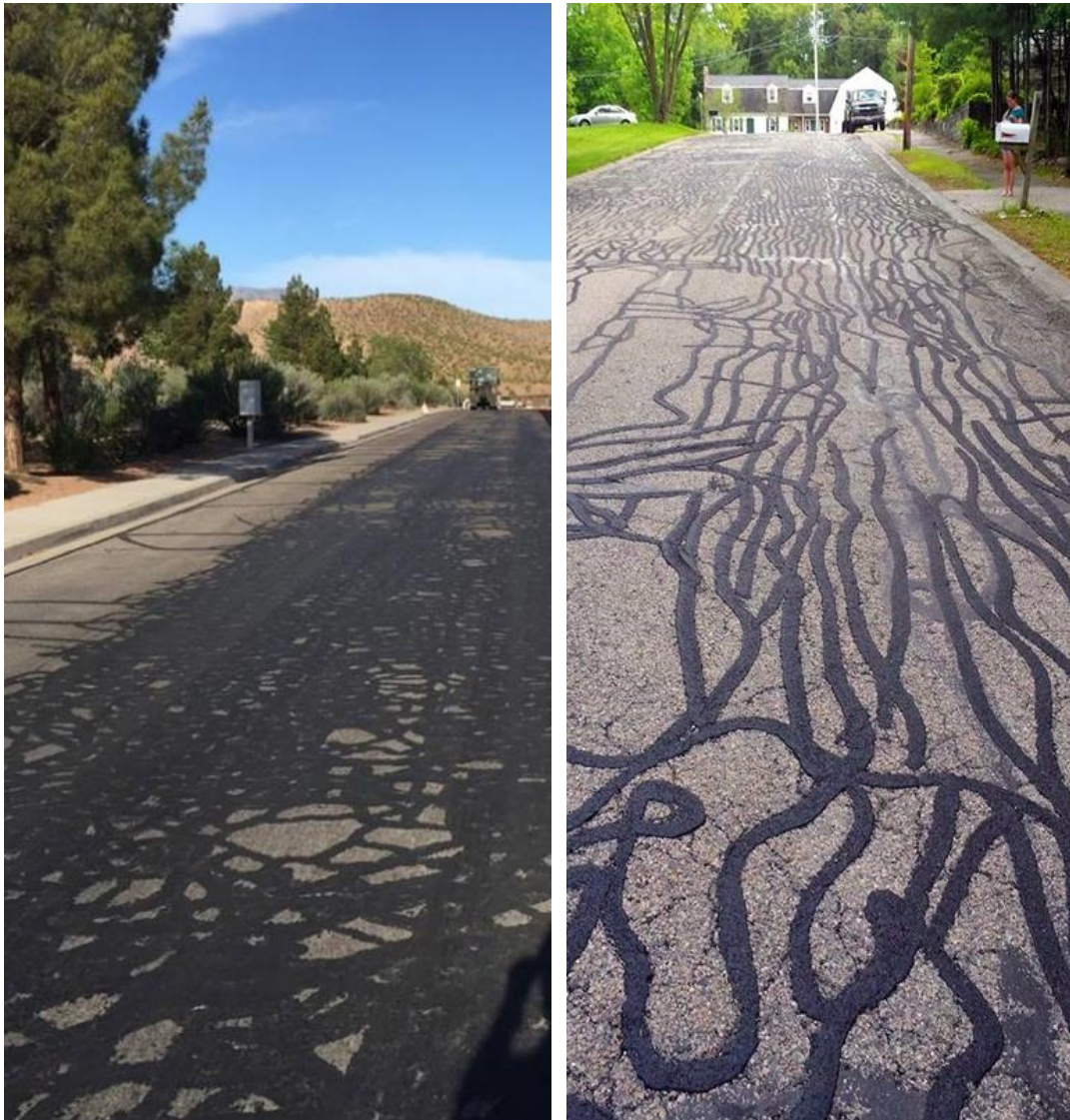
Figure 26. Improper Project Selection
