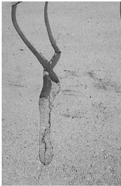
Figure 12. Sealant Peeling as Result of Improper Cleaning (Courtesy of Crafc0)
