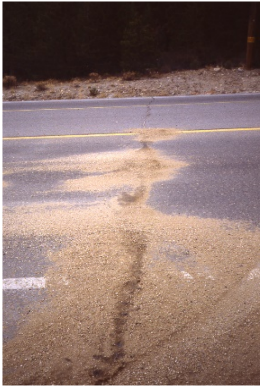
Figure 28. Excess Sand Must Be Removed Prior to Traffic
