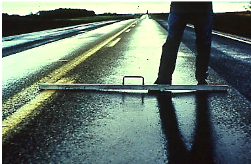
Figure 62. Rutting Requiring a Leveling Course Prior to Overlaying
