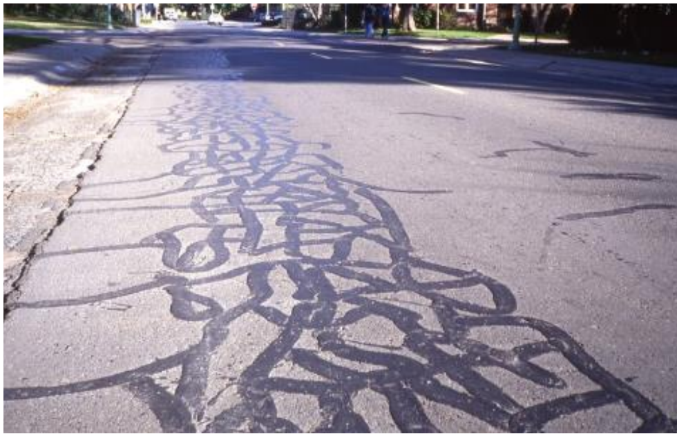
Figure 3. Attempt at Sealing Alligator Cracking
