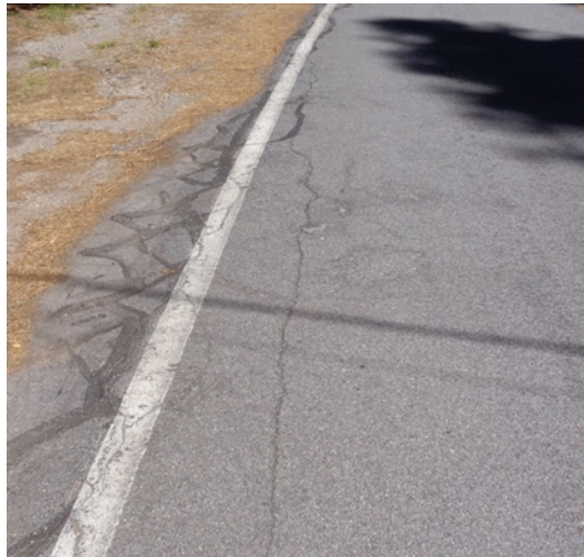
Figure 51. Example of Edge Cracking of a Pavement
