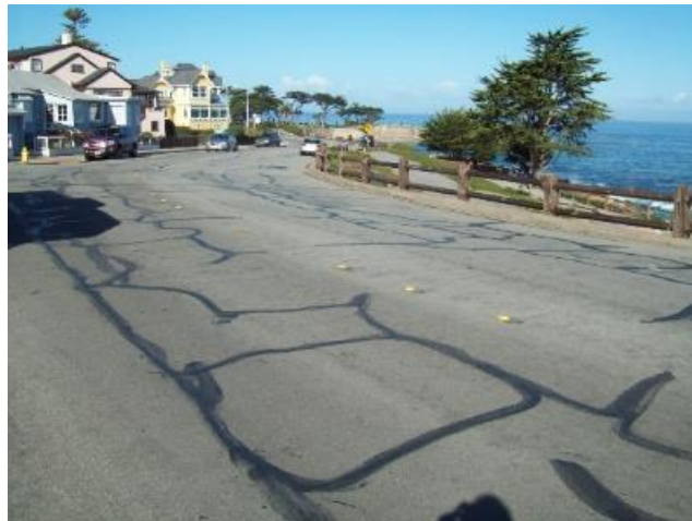
Figure 2. Ugly Crack Sealing on a Scenic Street
