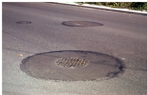
Figure 65. Manhole Iron Raised after Overlay
