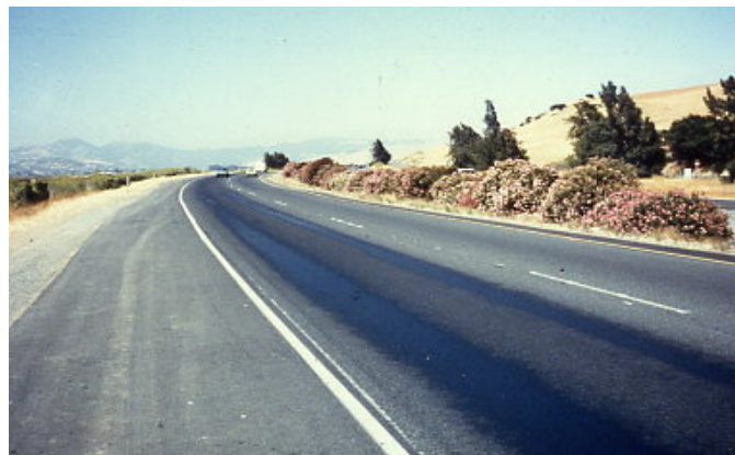
Figure 63. Chip Seal Placed over Rutted Pavement
