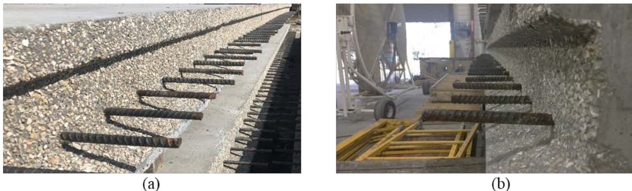
Figure 8.16: FIU-3 joint reinforcement length observations at (a) precast yard and (b) structures lab
