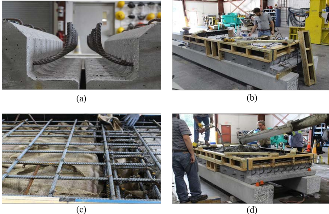
Figure 5.11: Construction of deck and joint in FSB: (a) adjacent FSBs with \frac{3}{4} " spacing, (b) CIP deck form construction, (c) slab and joint reinforcement, and (d) CIP deck pour
