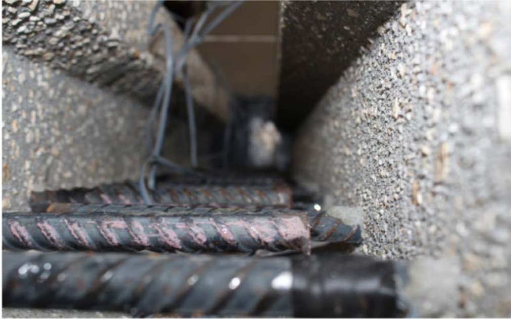
Figure 5.24: Transverse rebar misalignment observed in Alternate 2 joint specimen
