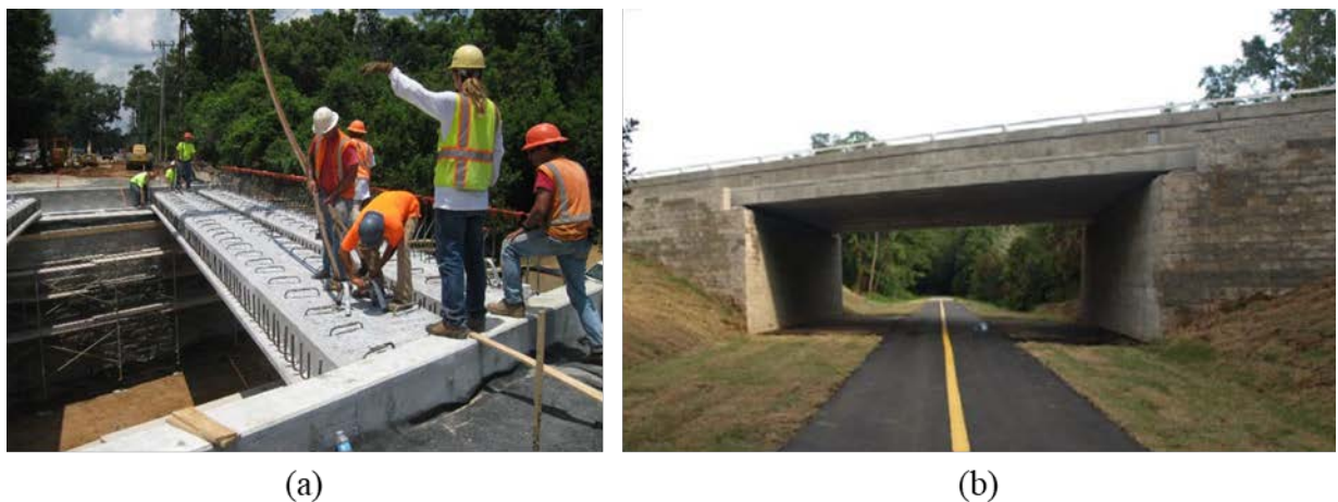
Figure 2.23: (a) Placement of FSBs adjacent to each other and (b) finished pilot project SR-373 [16]
