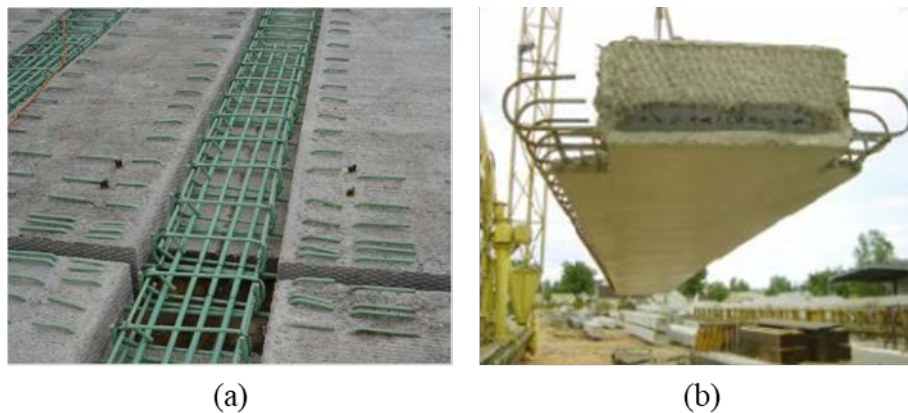
Figure 2.30: Additional reinforcement required in (a) transverse direction [25] and (b) extending from side of members [26]
