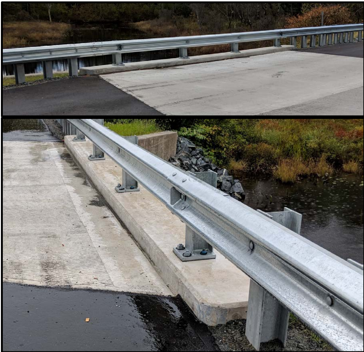
Figure 3: Example of a concrete bridge curb. This curb is approximately 29 ft. long and is located on NH 113 in Grantham, NH.
