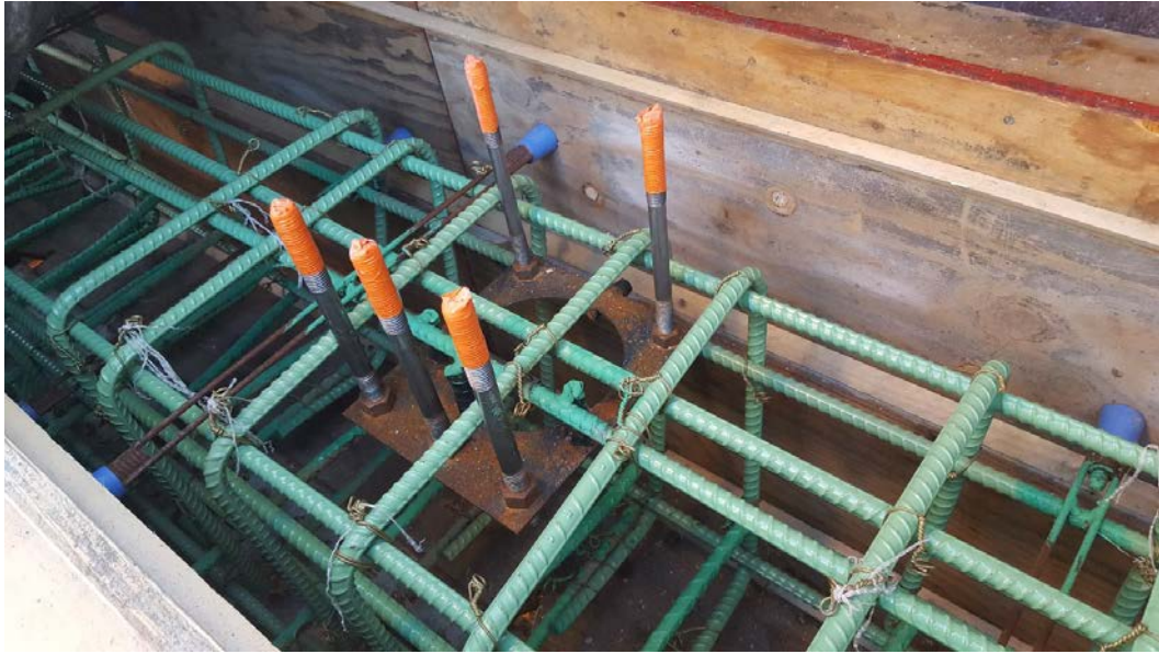
Figure 6: Guardrail anchorage and reinforcement in curb formwork. Tape on the top of the anchoring system keeps threads clean during concrete placement.
