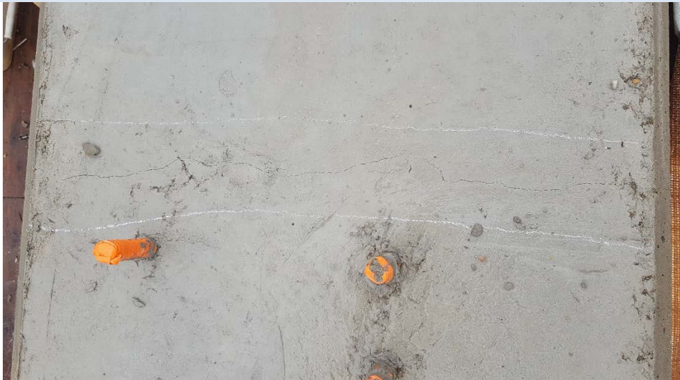
Figure 1: Crack in a bridge curb 5 days after placement.
