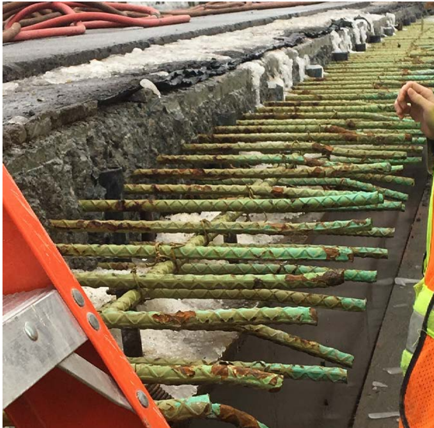
Figure 4: Exposed rebar extending out from a bridge deck after the former curb had been demolished.
