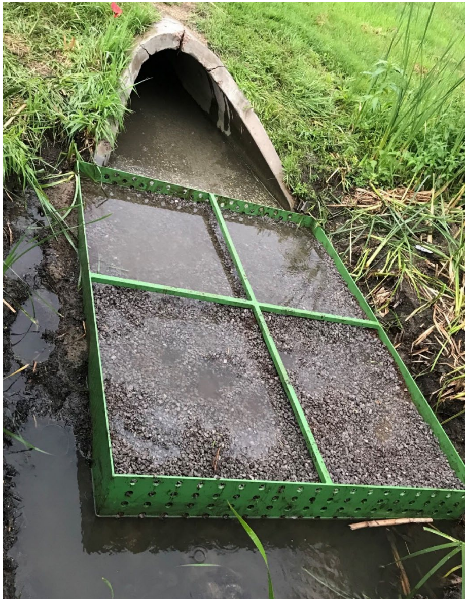
Figure 5.6 Field scale stormwater filter installed at a residential stormwater detention pond.
