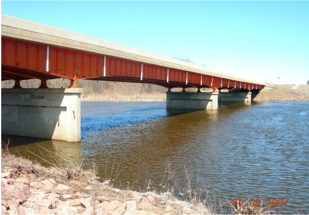
Figure 6.2 SD13 bridge from left bank facing along upstream face toward right bank The pier sets in the photograph are, from left to right, bents 4, 3, and 2. The photograph was taken by Francis Ting on April 6, 2007.
