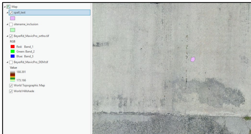
Figure 6.3.7: False positive for Beyer Rd bridge location used as the example. Output is a polygon shapefile with detected spalls. Adjust sensitivity higher to detect more potential spalls, lower to detect less false positives.
