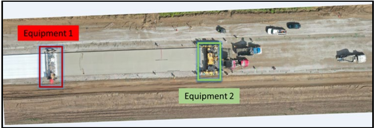
Figure 3.3.5: Image labeling example – MDOT I-496 Project (Samsami et al., 2021). Equipment can be identified in drone imagery/orthoimages using automated image processing packages available in MATLAB.
