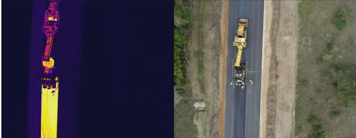
Figure 6.7.1: DJI RGB thermal image (left) and visual image (right) collected simultaneously by the Mavic 2 Enterprise Advanced during asphalt paving. The image on the left is an RGB representation of the thermal data captured by the M2EA’s thermal camera and does not contain true-temperature thermal information (made inaccessible by DJI for batch processing).
