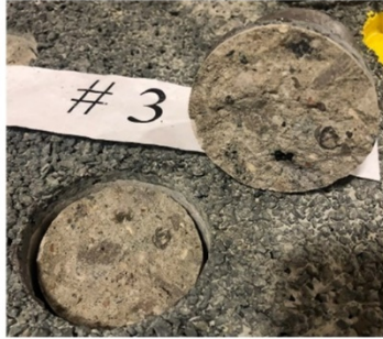
i) Failure in room temperature
