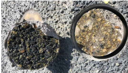
b) E1 epoxy overlay under outdoor summer exposure
