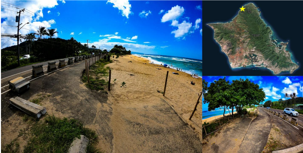
Figure 6-6 Bike path, beach parking, and road are eroding into the ocean at Sunset Beach
