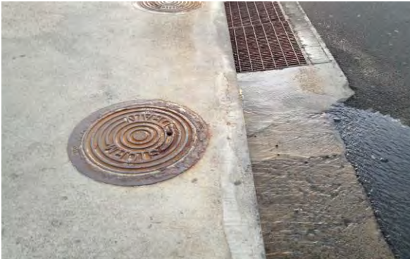
Figure 2: Waikiki storm drains backed up with sea water during a king tide event in April 2015. Photo credit: Wendy Meguro
