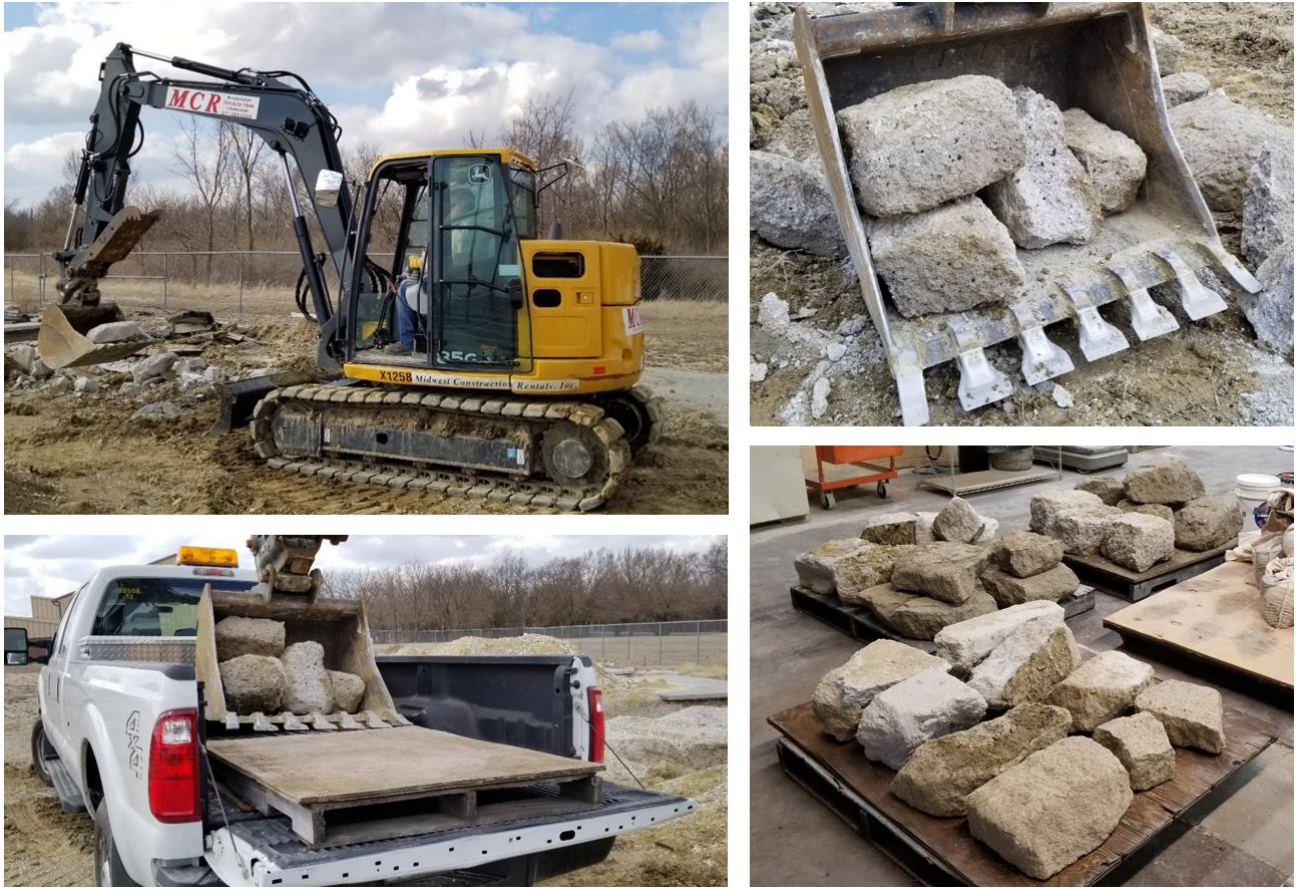
Figure 3.1. Extraction of stabilized QB materials from the test sections constructed for ICT-R27-168.
