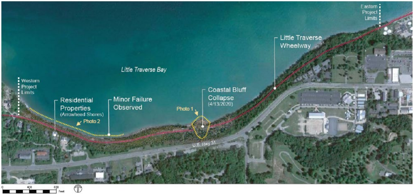
Figure 4-16. Aerial view of the catastrophic 2020 slope failure near western Petoskey, Michigan (from Baird, 2020)
