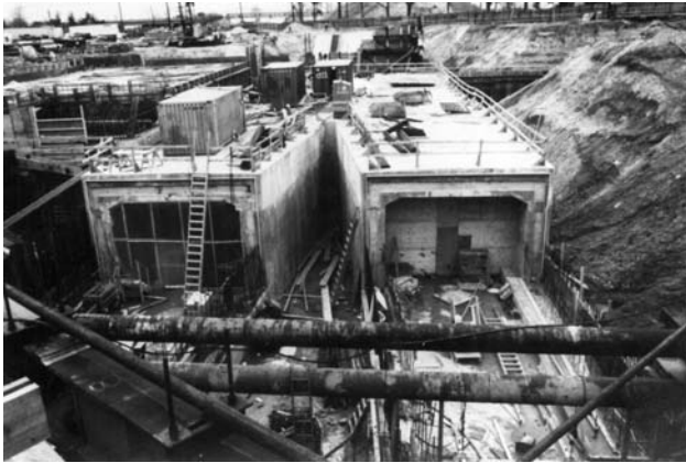
Tunnel construction for a Washington Metropolitan Area Transit Authority heavy rail line. Some tunnels are bored deep underground by special machines. This one employs the cut-and-cover method--digging a trench, building the tunnel, and then covering it up.
