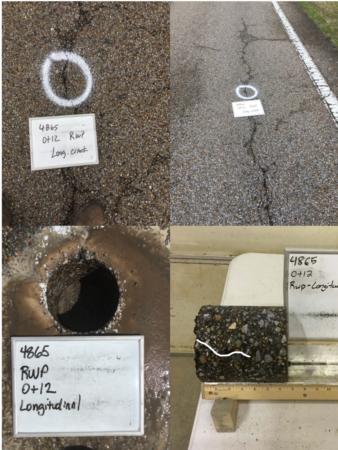
Figure 46: Pavement Surface and Core for Longitudinal Crack - Section 4865, Station 0+12
