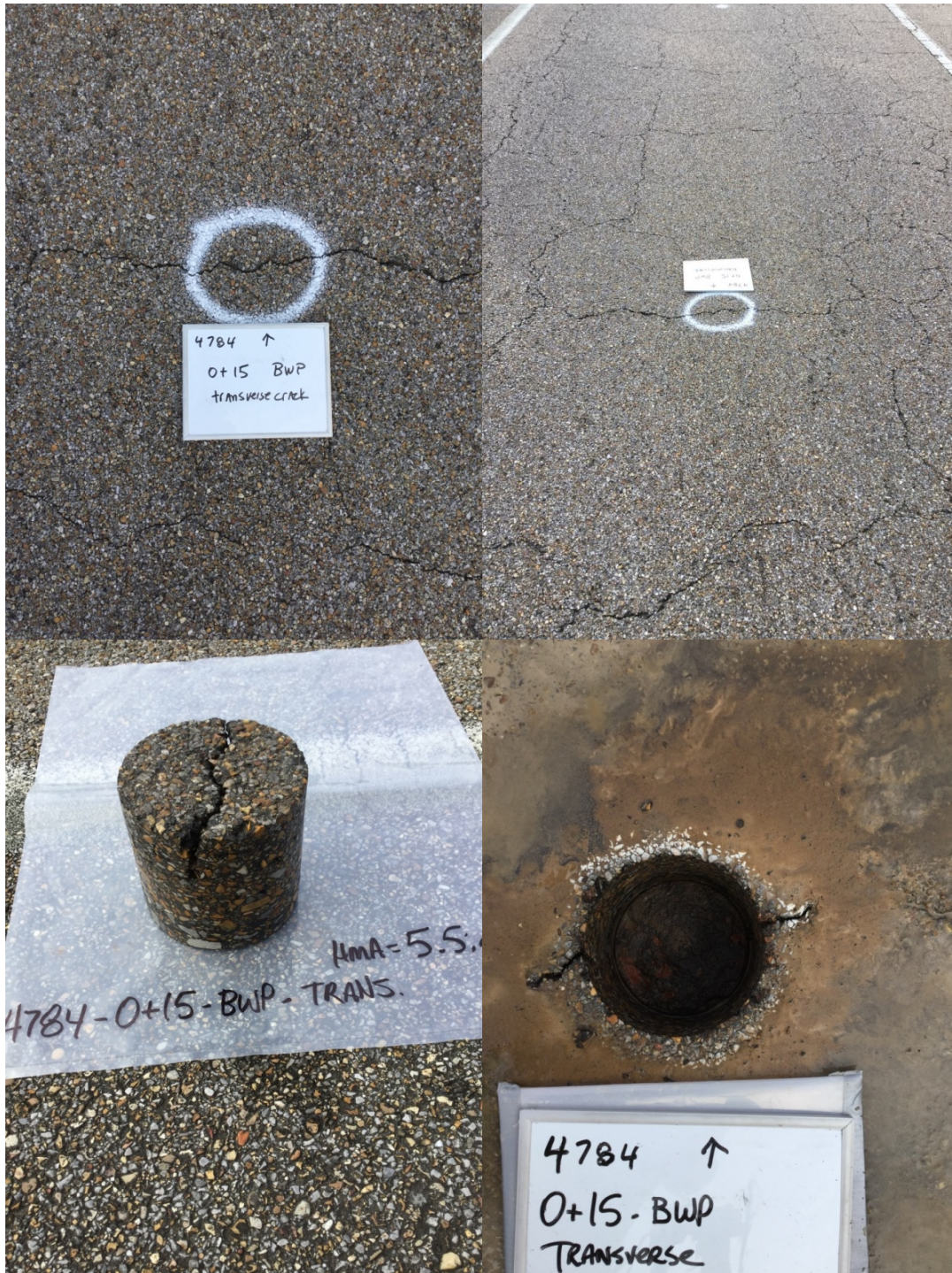
Figure 54: Pavement Surface and Core from Transverse Crack - Section 4784, Station 0+15
