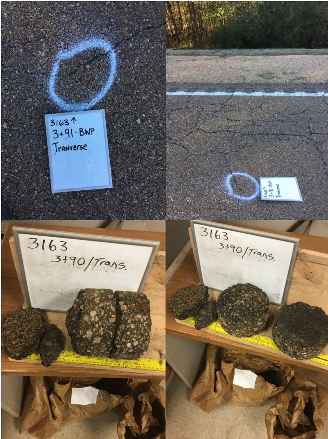
Figure 50: Pavement Surface and Core for Transverse Crack - Section 3163, Station 3+91
