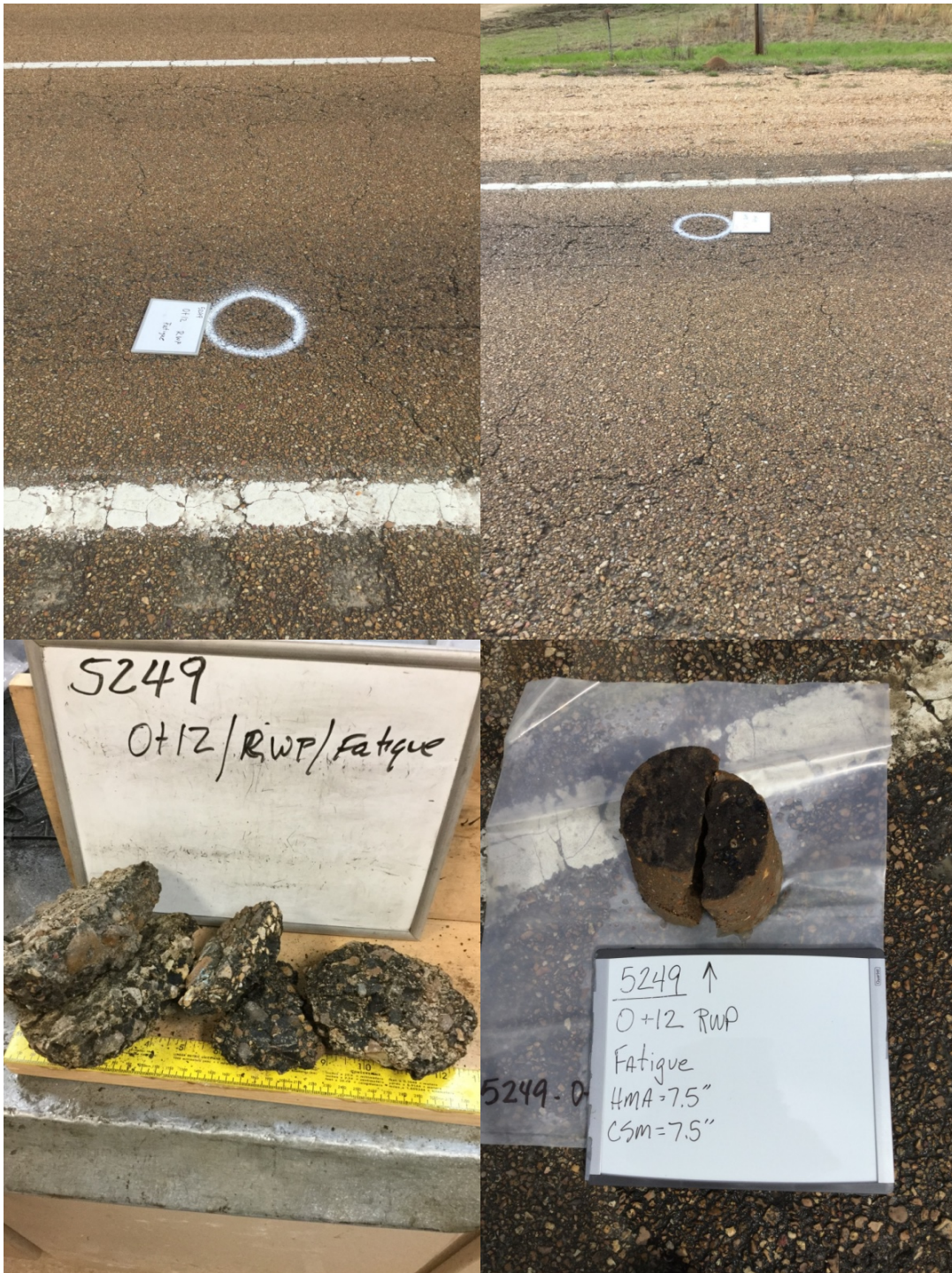
Figure 62: Pavement Surface and Core from Fatigue Crack - Section 5249, Station 0+12
