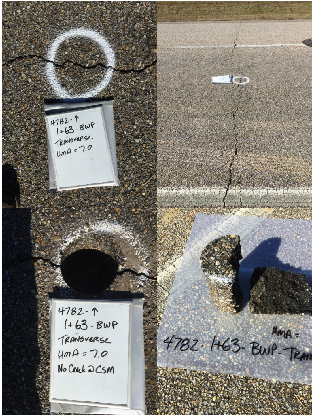
Figure 52: Pavement Surface and Core from Transverse Crack - Section 4782, Station 1+63
