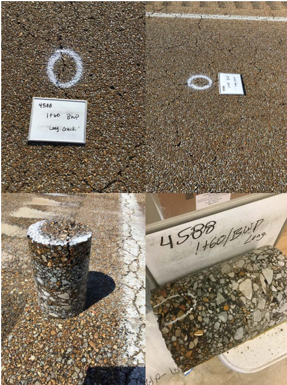
Figure 42: Pavement Surface and Core for Longitudinal Crack - Section 4588, Station 1+60
