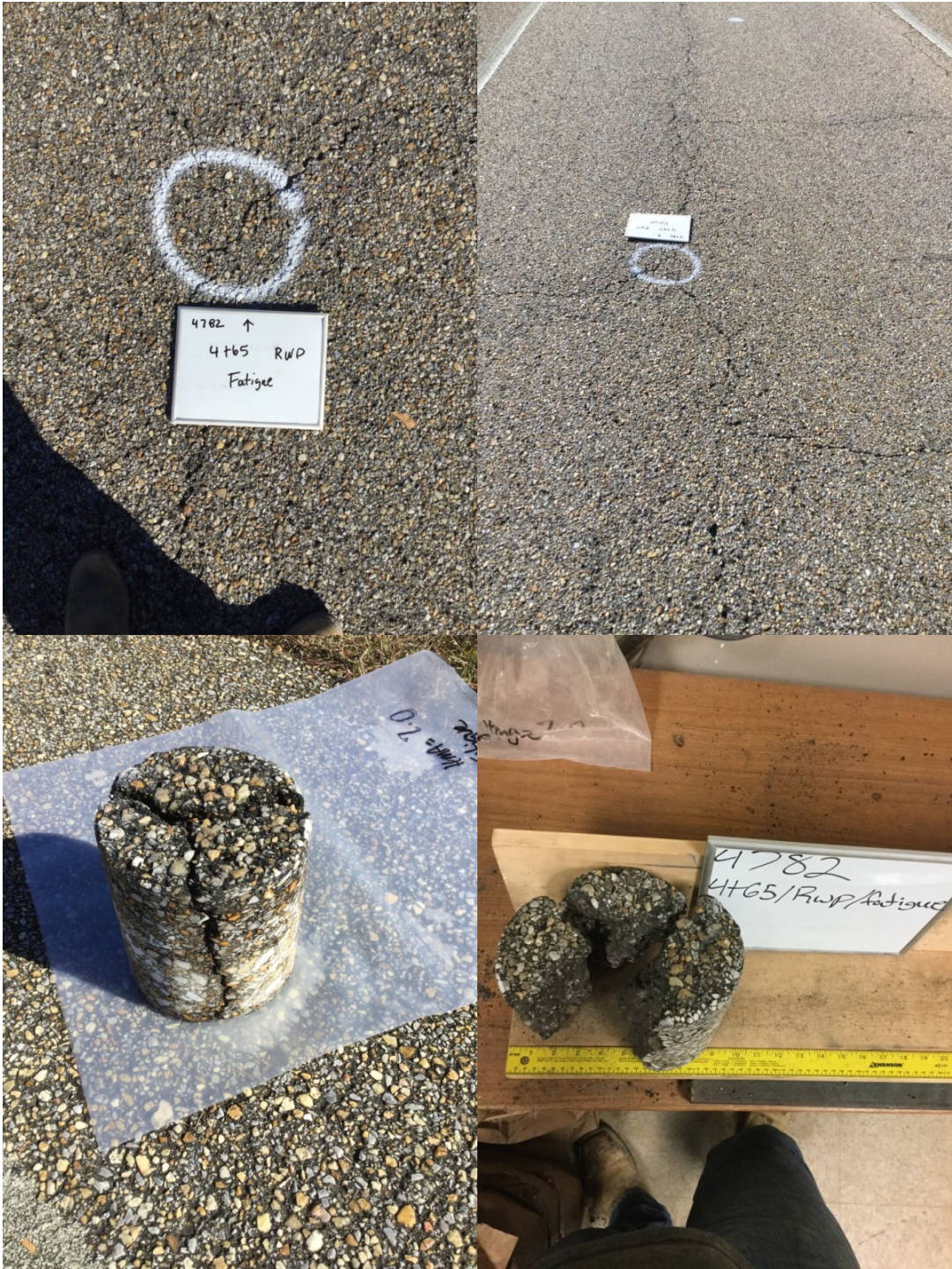
Figure 58: Pavement Surface and Core from Fatigue Cracks - Section 4782, Station 4+65
