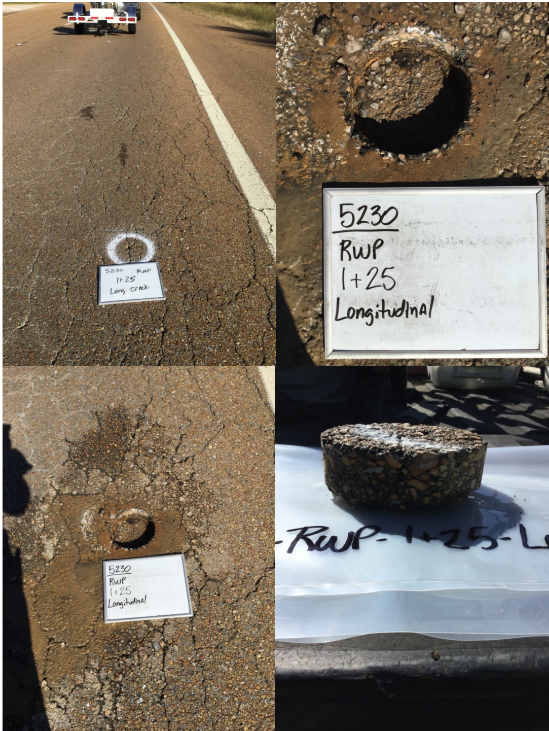
Figure 60: Pavement Surface and Core from Fatigue Crack - Section 5230, Station 1+25
