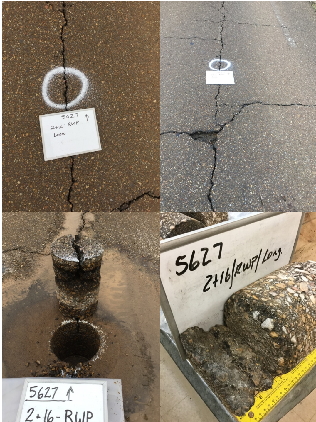
Figure 48: Pavement Surface and Core for Longitudinal Crack - Section 4865, Station 2+16
