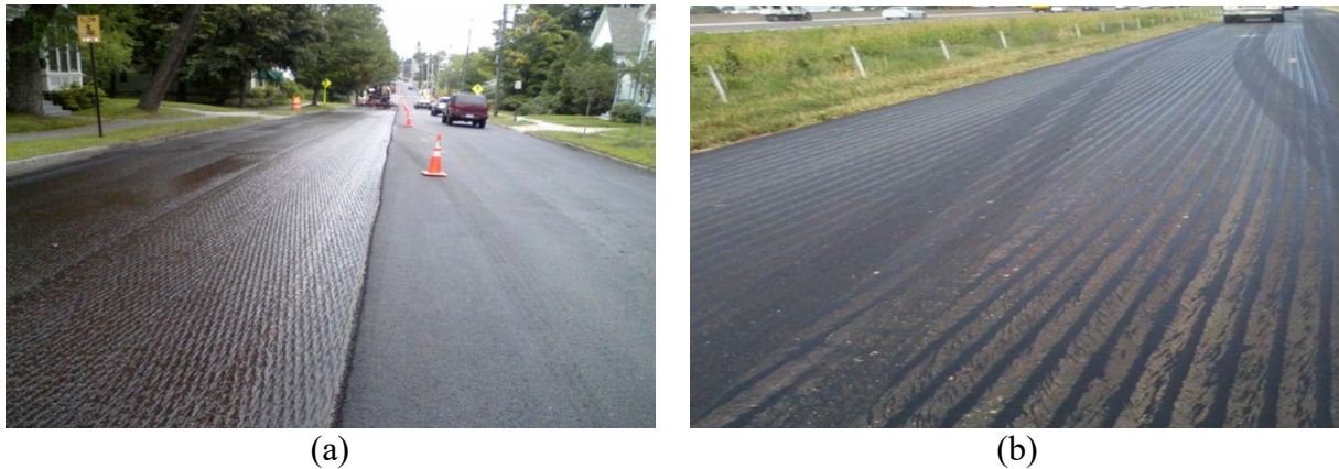
Figure 2.9: Tack coat application uniformity (a) Acceptable tack coat application uniformity (uniform), and (b) unacceptable tack coat application uniformity (non-uniform).
