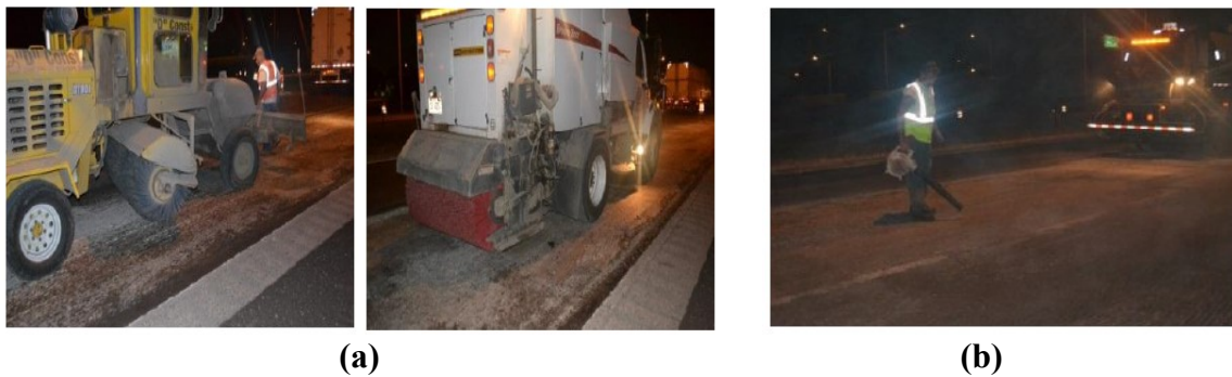
Figure 2.10: Cleaning methods (a) Sweeping and vacuuming and (b) air blasting (Al-Qadi 2012b).
