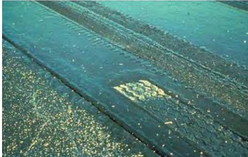
Figure 2.5: Excessive tack coat application (Mohammad et al. 2012).
