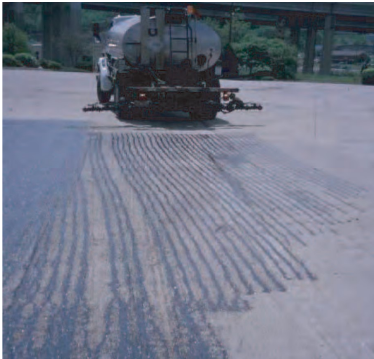
Figure 2.30: Tack coat streaking due to clogged nozzles (Mohammad et al. 2012).
