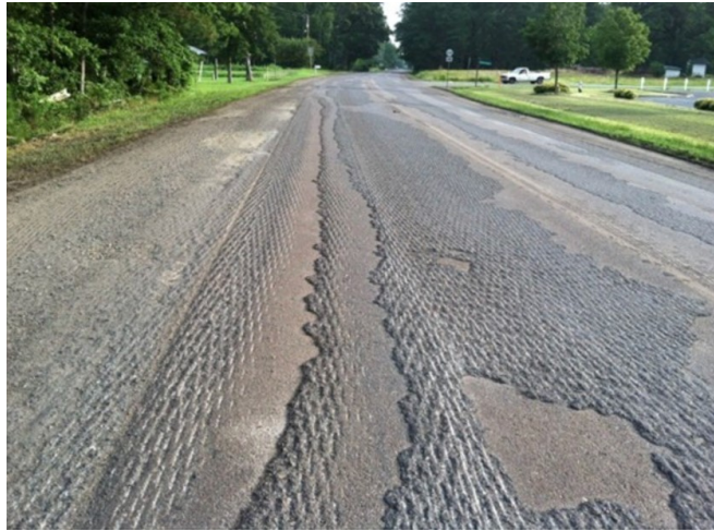
Figure 2.8: Scabbing of existing pavement after milling (Shiells 2015).
