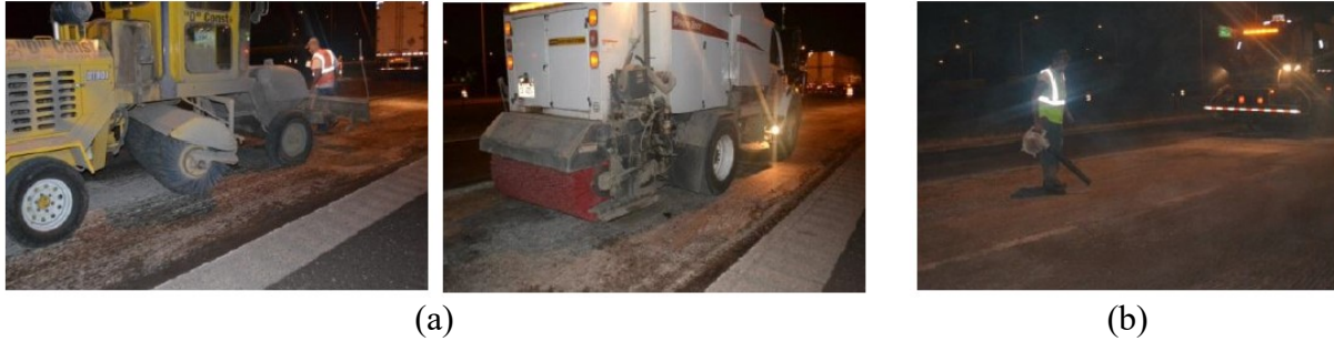
Figure 4.2. Common field cleaning methods: (a) Sweeping and vacuuming and (b) air blasting (Al-Qadi et al. 2012).
