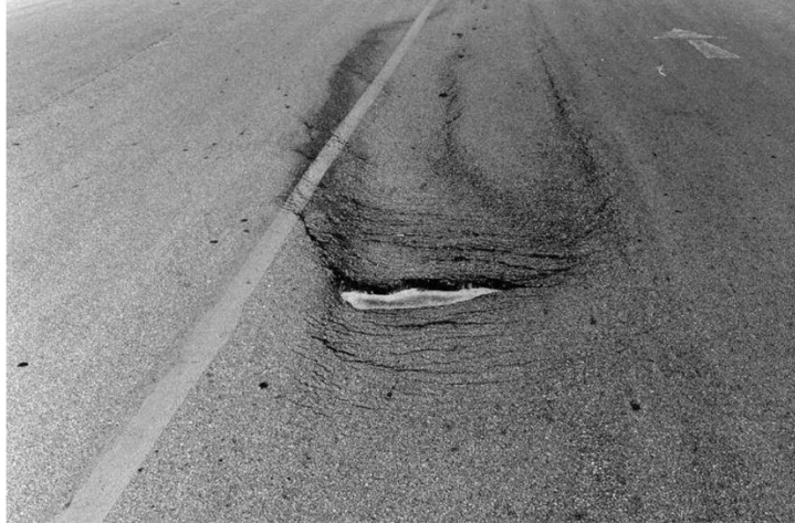
Figure 2.2. Slippage cracking caused by excessive tack coat (Al-Qadi et al. 2012b).
