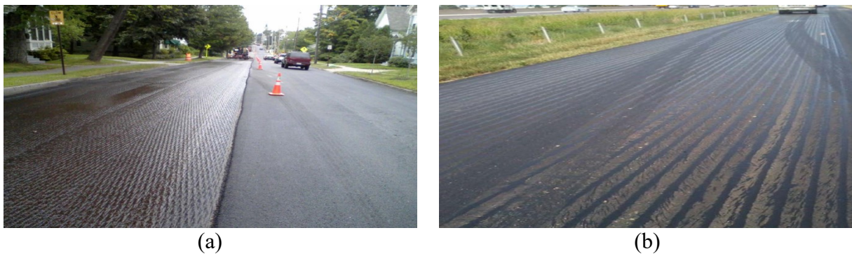
Figure 4.4: Tack coat application uniformity: (a) Acceptable tack coat application uniformity, and (b) unacceptable tack coat application uniformity (streaking) (FHWA 2016).
