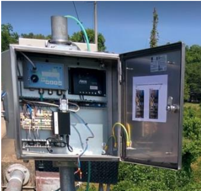
Figure 2-3 Interior of the gage electronics box
