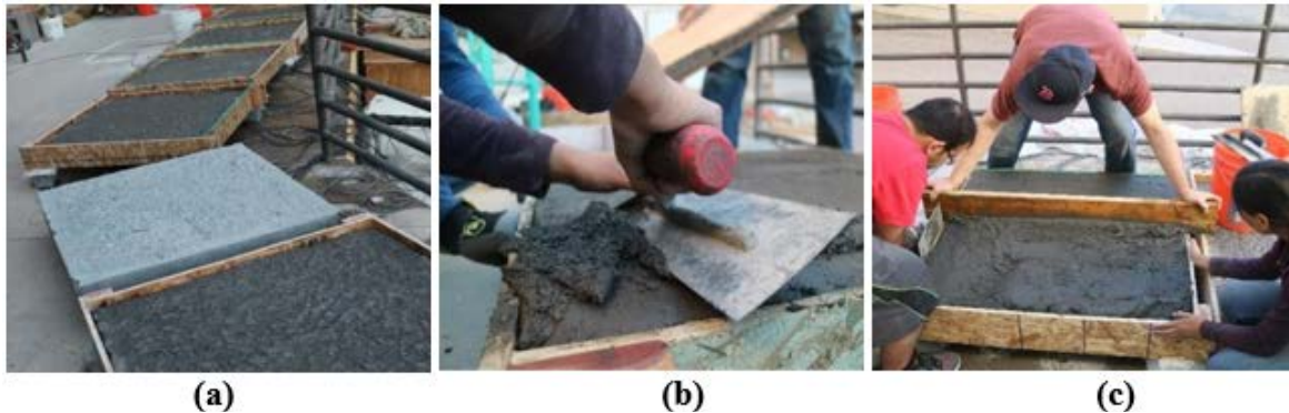
Figure 15. Preparation of UHPC overlay: (a) saturated rough surface with exposed aggregates before UHPC application, (b) workable consistency of UHPC mixture, and (c) tools used during the surface finishing of the overlay.
