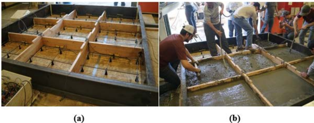
Figure 14. Slab construction: (a) formwork and sensors and (b) placement of NSC substrate.
