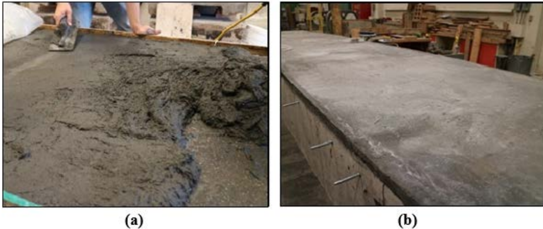
Figure 20. UHPC overlay on girder H-PS-C-300-R-UO (a) during placement and (b) prior to testing.
